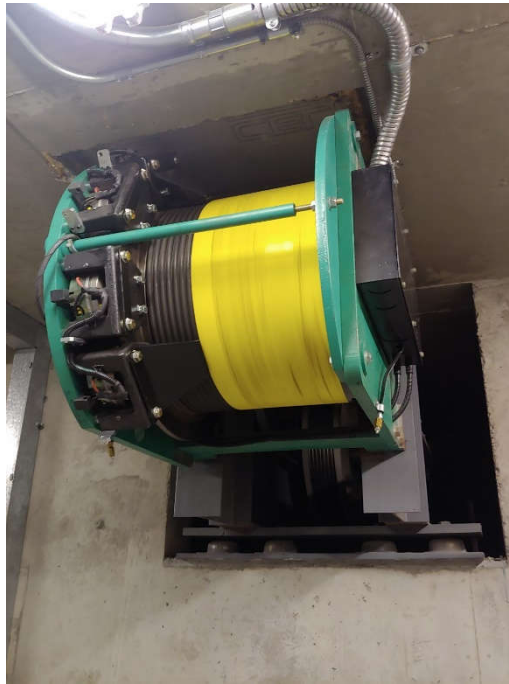
Photo 1: Elevator hoist machine
