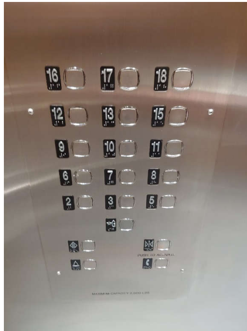
Photo 6: Elevator car operating panel
