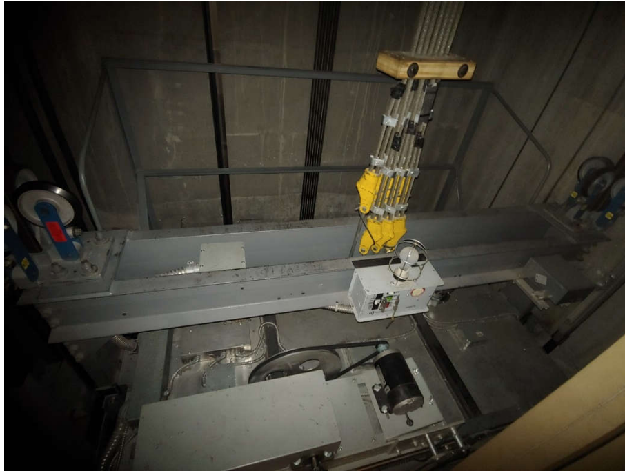
Photo 3: Elevator car top
