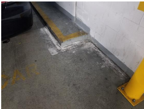
Photo C.- Efflorescence in concrete block firewall and concrete floor due to water ingress outside the emergency generator room
