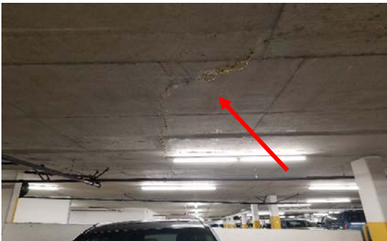
Photo D.- Crack possibly injected with polyurethane foam located beside the ramp which ends at P1
