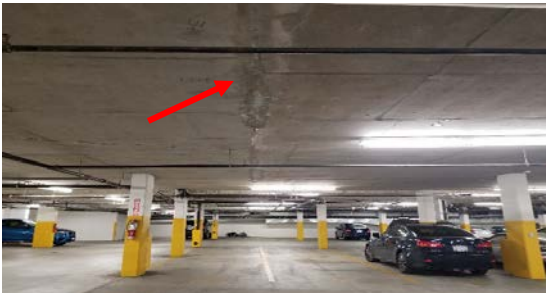
Photo C.- Notorious water ingress from the commercial parking level towards P1 level
