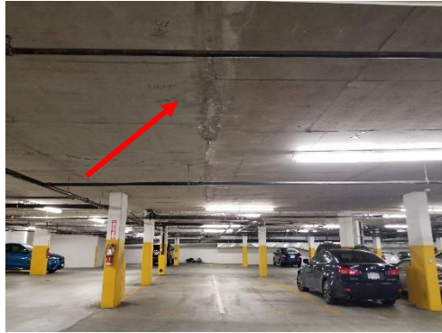
Photo C.- Notorious water ingress from the commercial parking level towards P1 level
