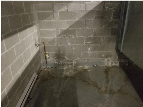
Photo B.- Efflorescence in concrete block firewall due to water ingress in the emergency generator room
