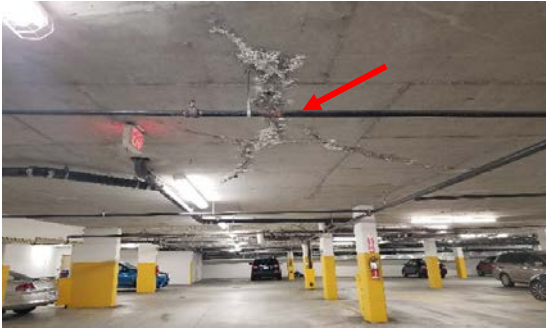
Photo B.- Notorious water ingress from the commercial parking level towards P1 level
