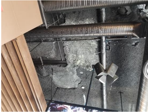
Photo A.- Exposed concrete slab in the ceiling of Urban Gate Restaurant
