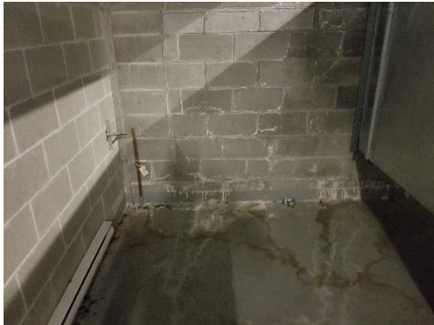
Photo B.- Efflorescence in concrete block firewall due to water ingress in the emergency generator room
