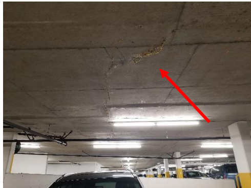
Photo D.- Crack possibly injected with polyurethane foam located beside the ramp which ends at P1
