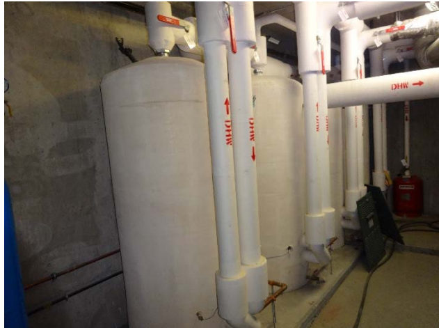
Hot water tanks
