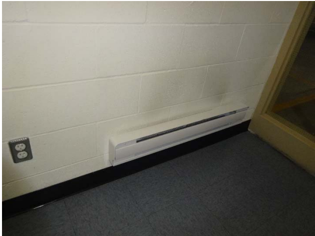
Electric baseboard heater on corridor
