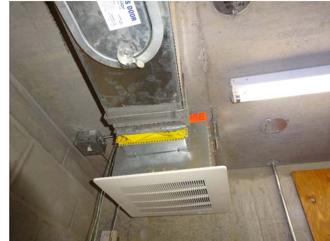
Exhaust fan in service room
