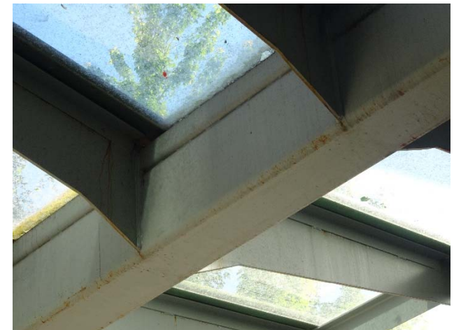
Corrosion spots on metal frame
