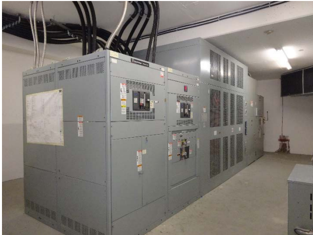
High voltage substation
