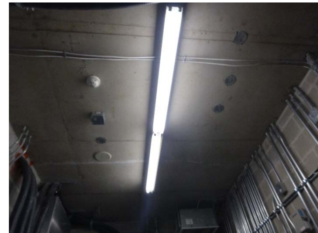
Light fixture in service room
