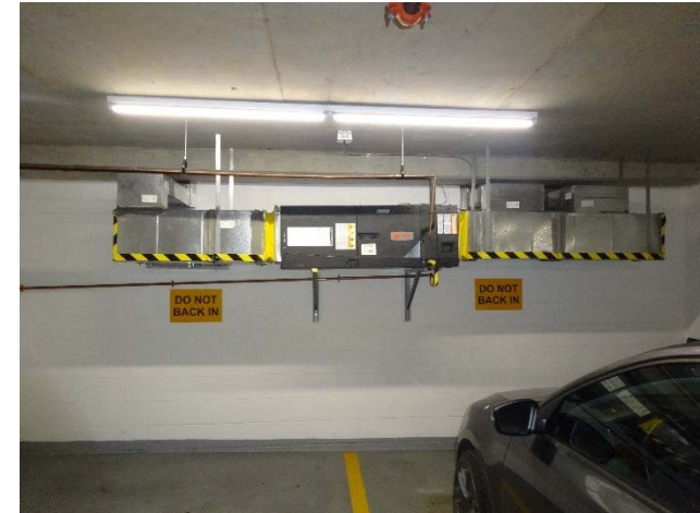
Transfer air unit
