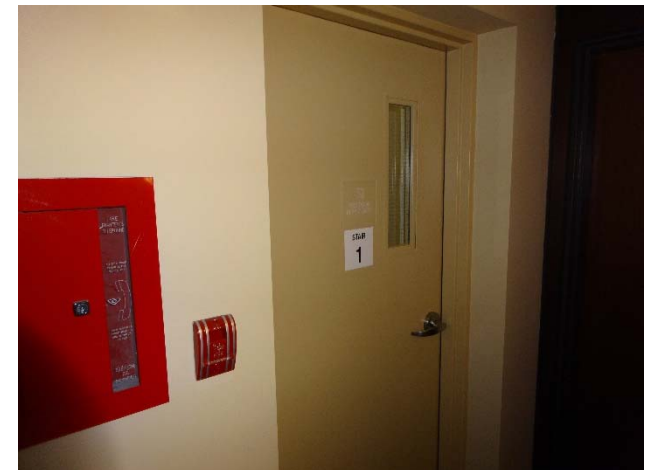
Emergency telephone both and pull station
