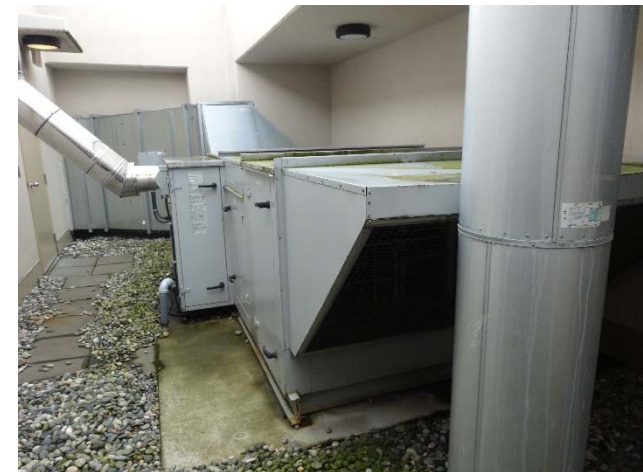
Make up air unit
