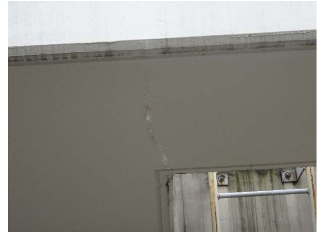
Crack extended through the entire thickness of the concrete canopy. Here view from underside.
