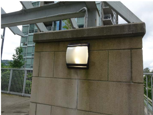
Light fixture on column
