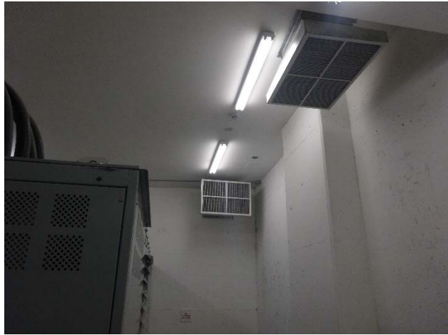
A/C fans in High Voltage room
