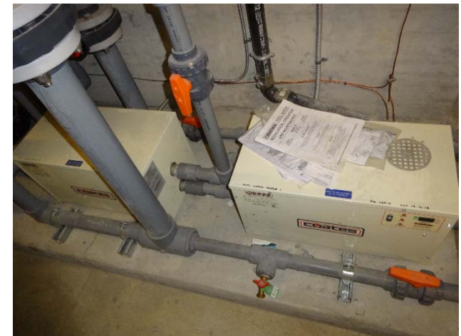
Water feature heaters
