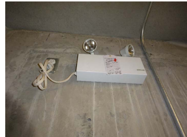
Emergency light fixtures with battery pack
