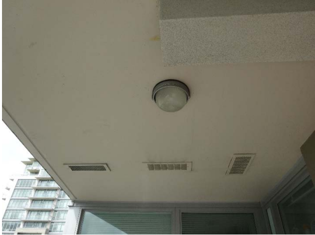
Light fixture on balcony
