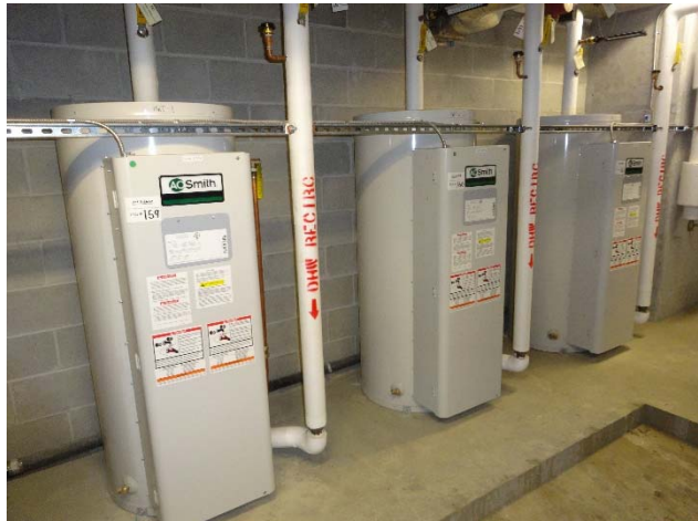
Hot water tanks
