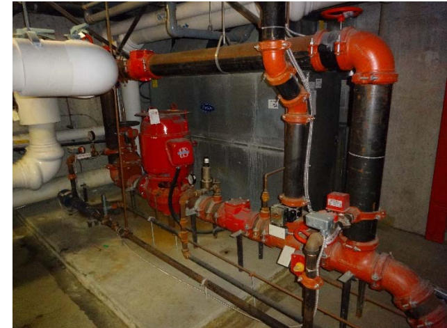
Fire pump assembly
