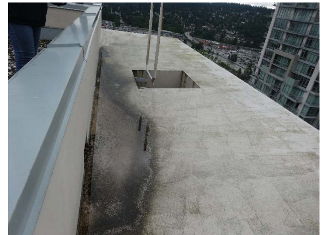
Water ponding due to missing storm drains at the lowest point.
