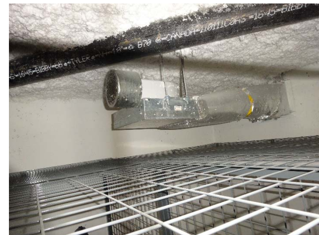
Exhaust fan in storage room
