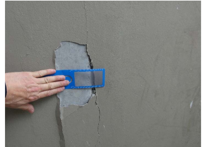
Crack and spalled coating
