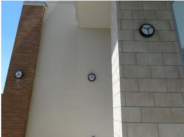
Light fixture on building facade
