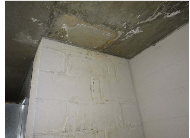
Cracks with efflorescence and water stains
