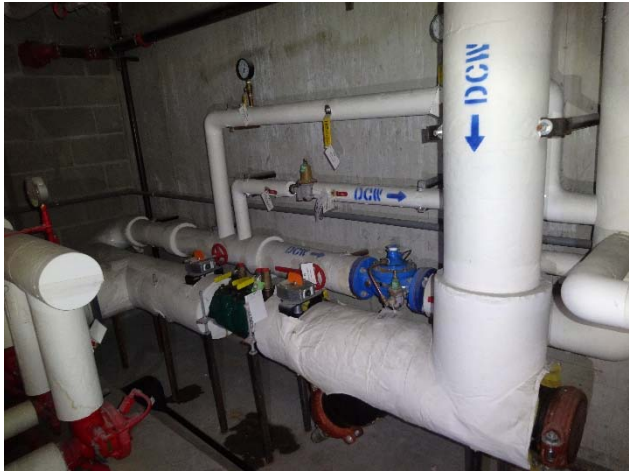
Water entry station
