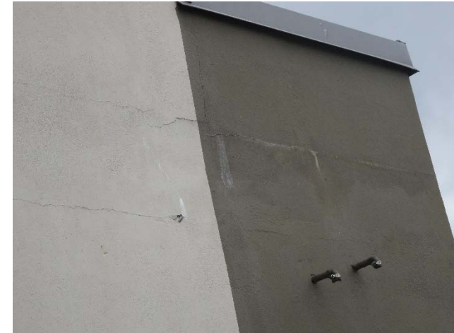
Cracks along cold joints
