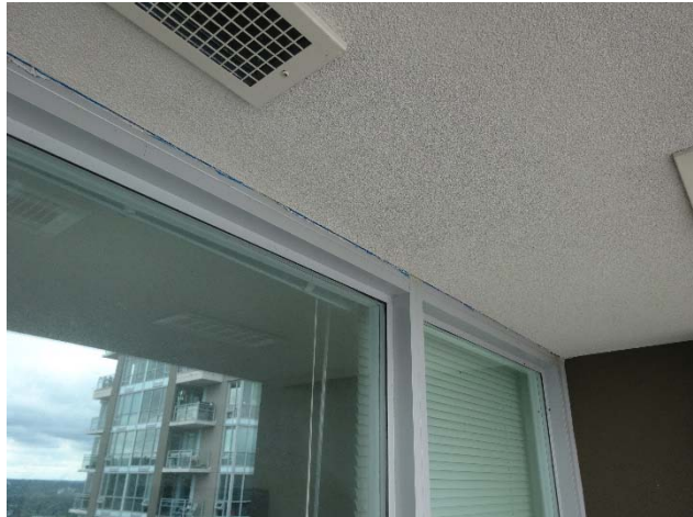
Missing caulking at unit #3208
