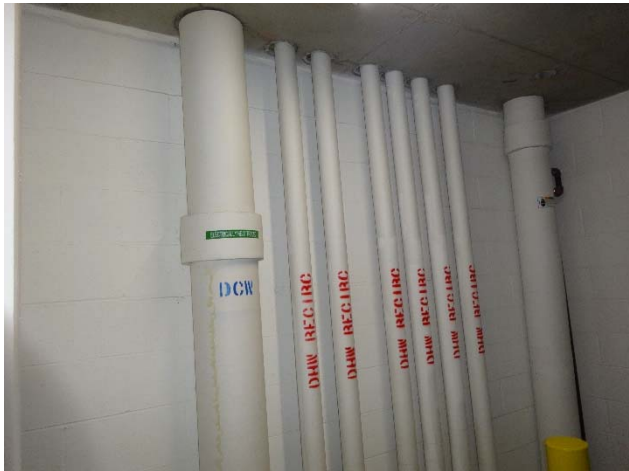
Water distribution piping
