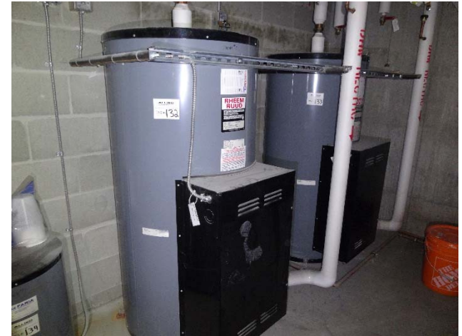
Electric water heaters
