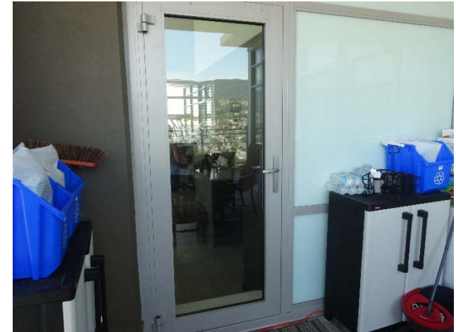
Swinging door on terrace
