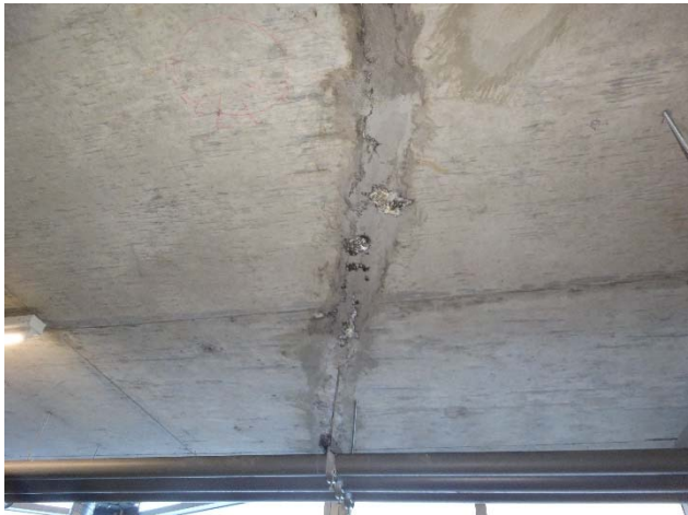
Repaired crack with water infiltration recurrence that denotes failure of the waterproofing membrane in the area
