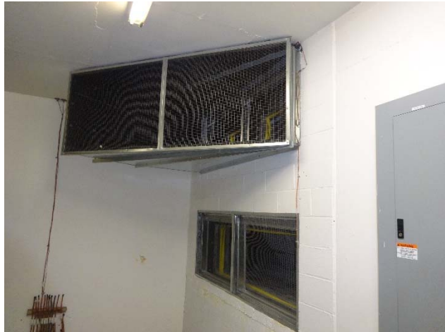
A/C fans in High Voltage room
