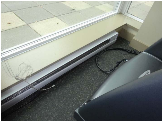
Electric baseboard heater in exercise room
