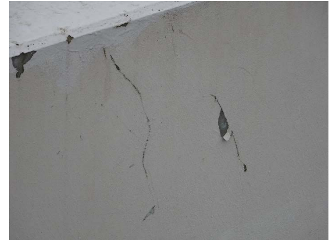
Scratched and peeling paint
