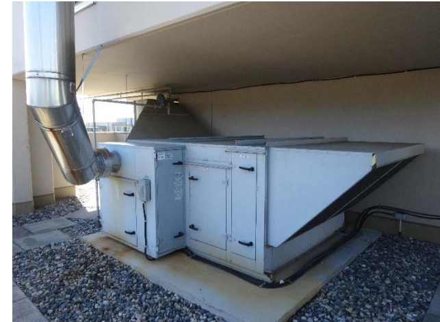
Make up air unit
