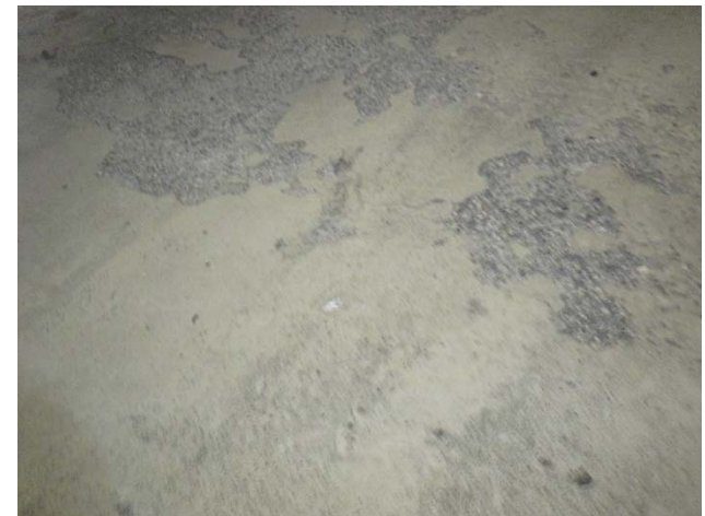
Scaled concrete surface with delaminated coating on parkade floor
