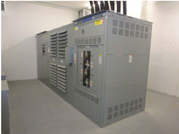
High voltage substation
