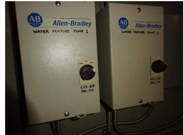
Water feature pumps
