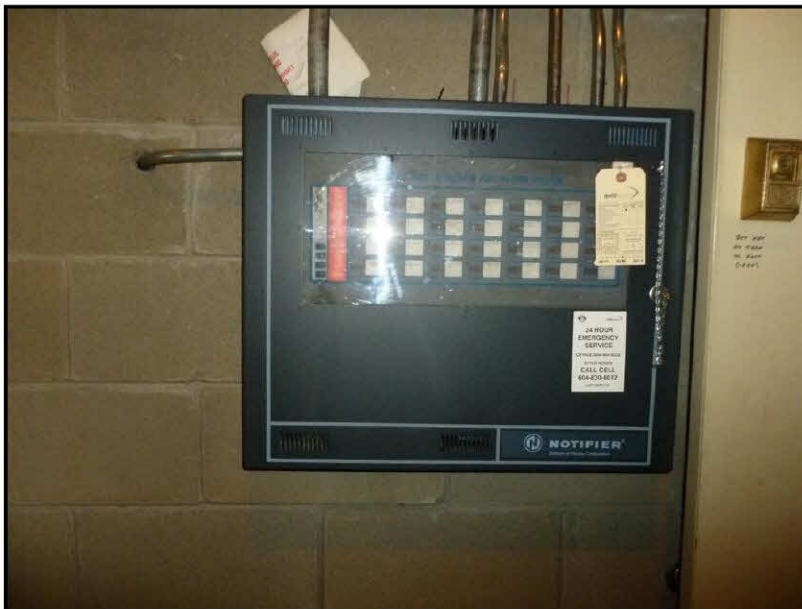
Photo No. 20: Typical fire alarm panel
