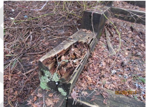
Observed existing wood deterioration in timber edging beside steps.
