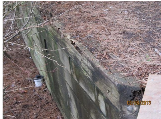
Observed existing wood deterioration in timber retaining wall.
