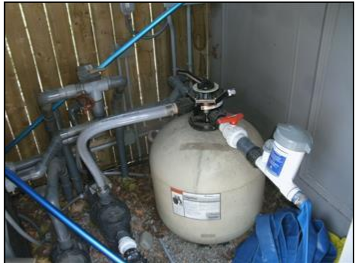
Pump and filter
