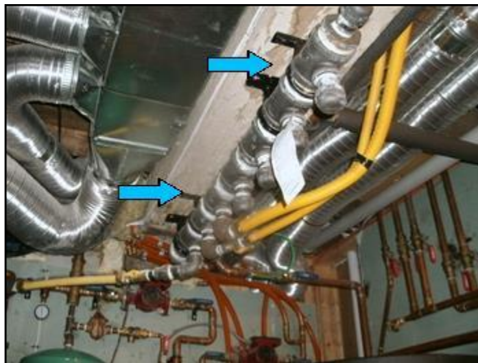
Large natural gas manifold
