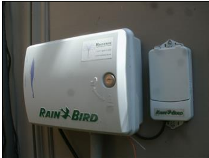
Irrigation System Controller
