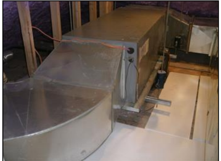
Air handler in 3rd floor knee wall.
