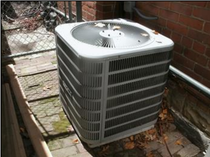
Independent system - air cooled
