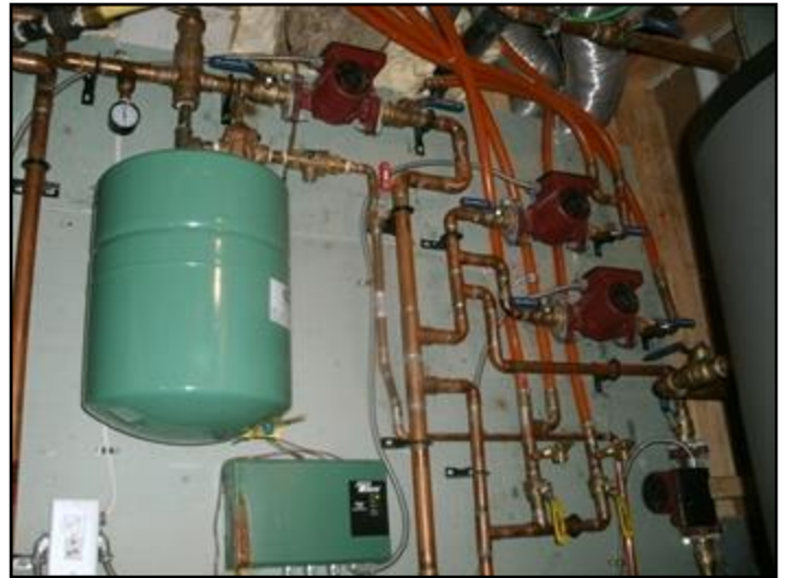
Expansion tank & circulation pumps
