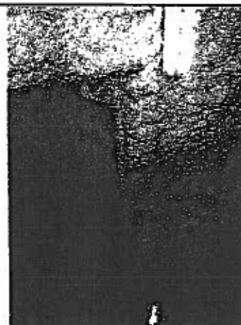
Photo 52: Parking garage: Note evidence of water leaking through the spray foam insulation.
