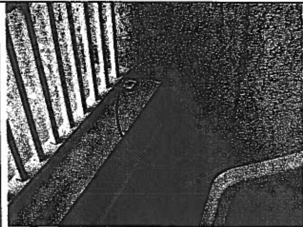
Photo 51: Unit #208 South facing balcony East wall: note lack of end dam on cap flashing and water staining.
