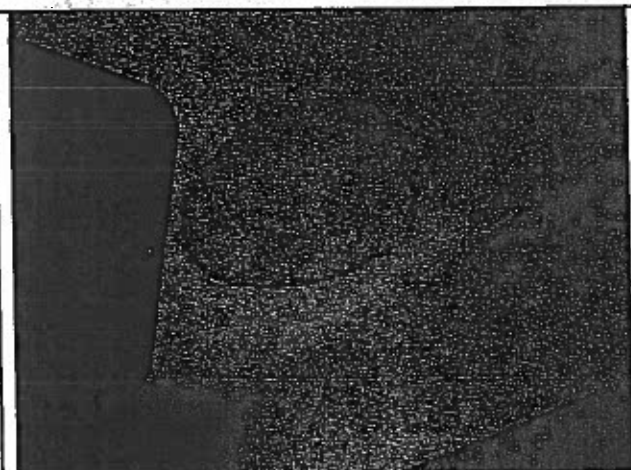
Photo 21: Unit #206: note water stains on ceiling. Evidence of water ingress from above.
