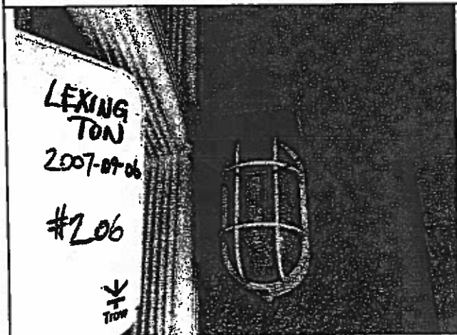
Photo 23: Unit #206 Level 3 balcony: note proximity of vent to light fixture. Warm moist air will rust the light fixture.
