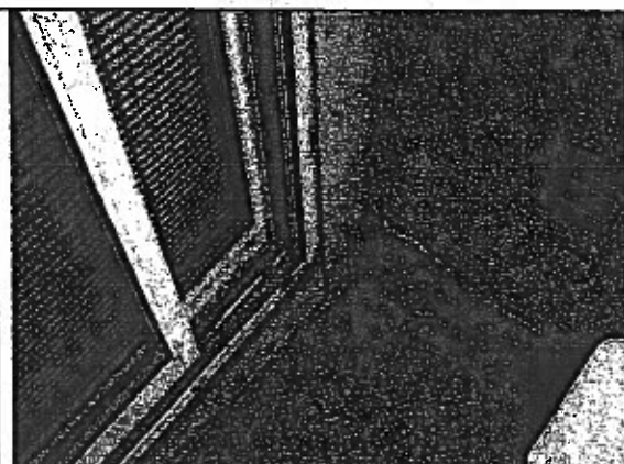
Photo 48: Unit #208 South elevation balcony: note high water mark on stucco wall. This indicates periodic water ponding and capillary saturation of adjoining stucco.
