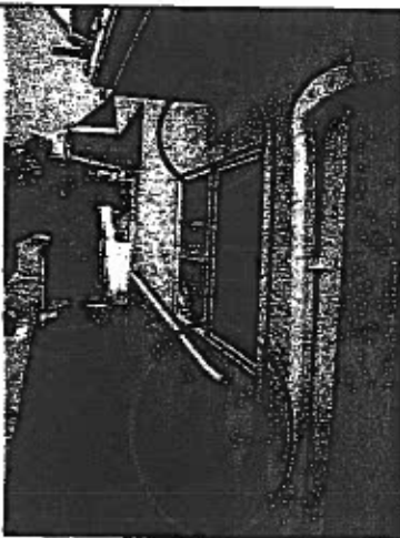
Photo 35: North elevation exterior walkway outside Unit #307: note water staining above and below window.
