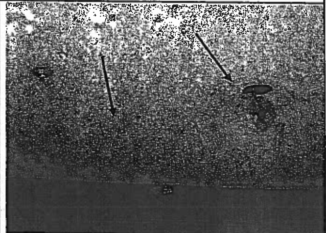
Photo 34: Unit #202 master bedroom: note water stains on ceiling.
