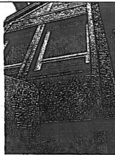
Photo 44: Unit #212 Level 3 East elevation: has been renovated in the past to be a "rain screen" look-alike.
