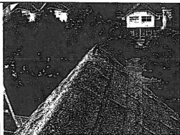
Photo 3: Deteriorated shingles at ridge.
