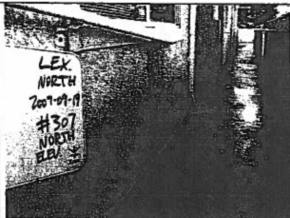
Photo 38: North elevation exterior walkway outside Unit #307: note water ponding along walkway.
