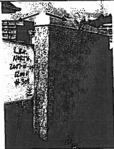
Photo 57: Unit #309 roof deck privacy wall is not adequately secured. It moves when little pressure is applied to top (see arrows).
