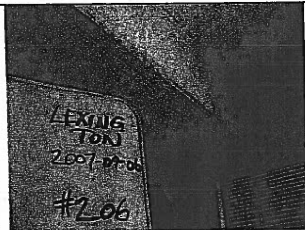
Photo 22: Unit #206: note water stains on ceiling. Evidence of water ingress from above.
