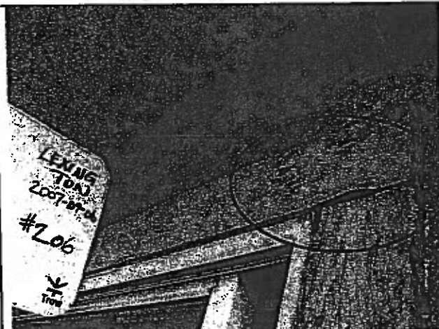
Photo 24: Unit #206 Level 3 balcony: deteriorated wood trim at sliding glass door.
