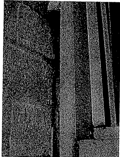
206 Discolouration behind sealant
