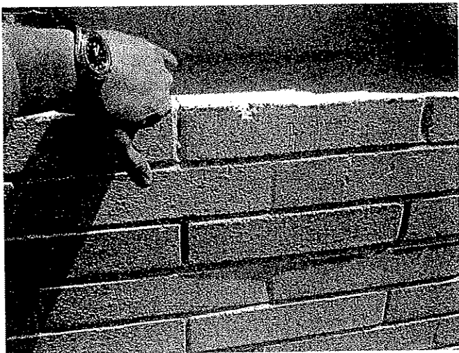
812 Mortar droppings filling cavity in the bottom three
