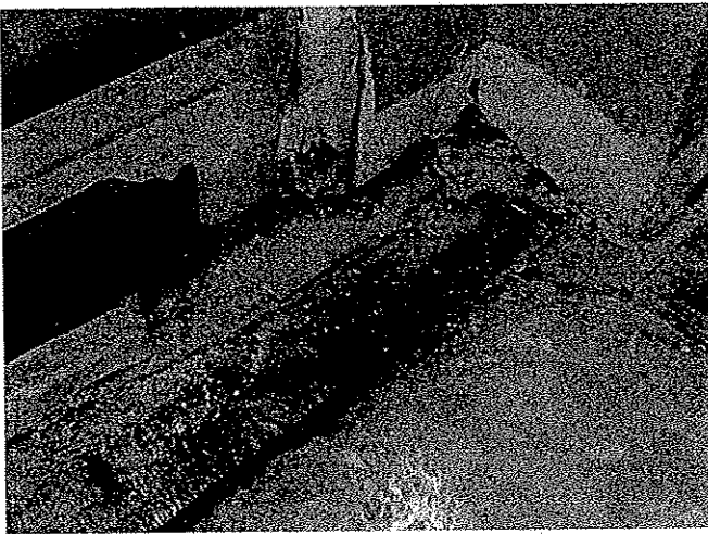
103 1608 Moisture damage at window sill, south east
