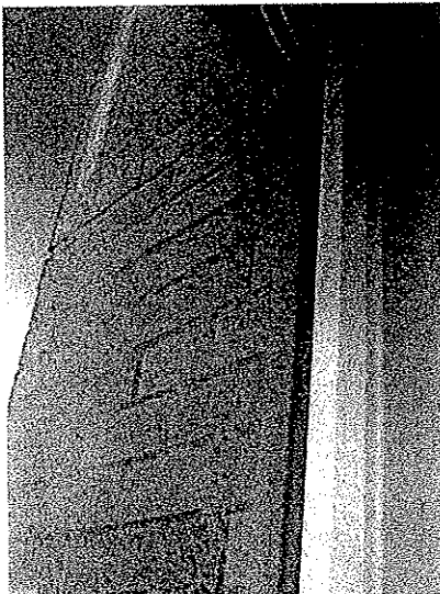
105 1608 Further staining at window adjacent to
