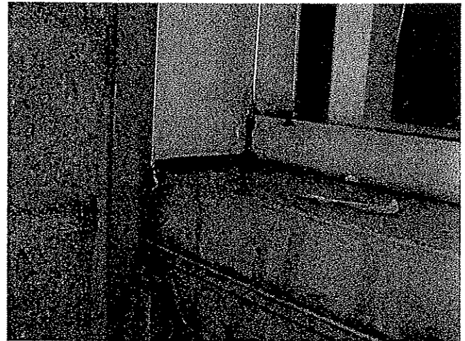
212 Water accumulation at window frame
