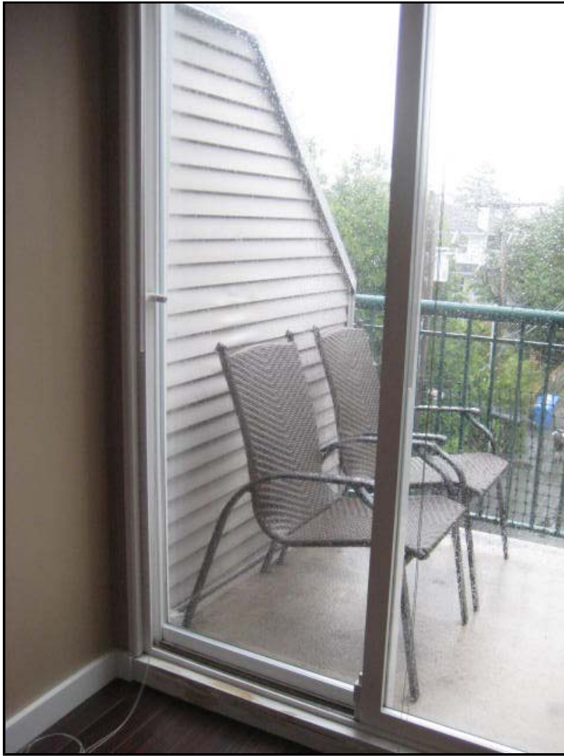
Photo No. 10: Suite 416 Sliding Door Note: Stained interior finishes below door.
