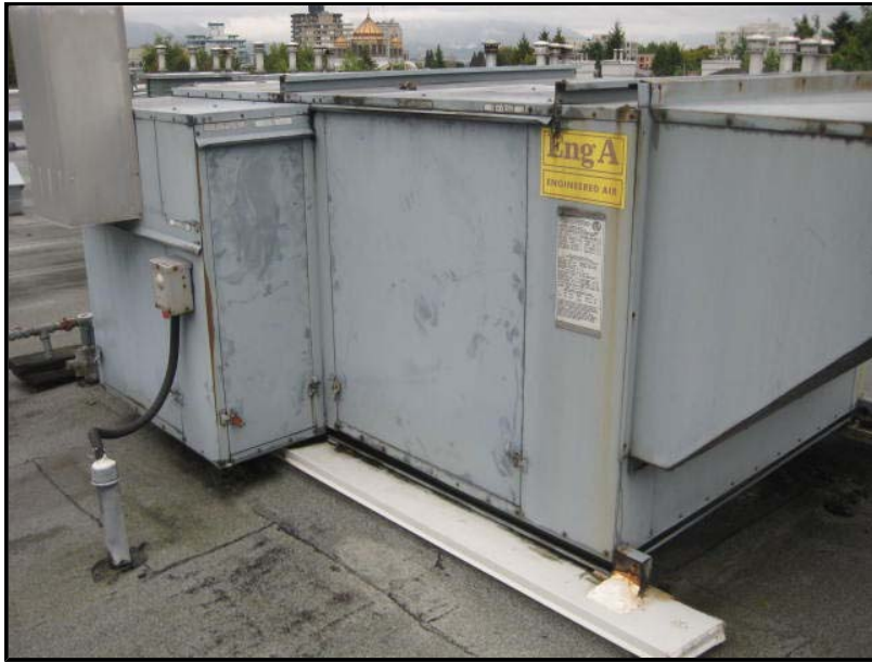
Photo No. 17: Roof Top Makeup Air Unit
