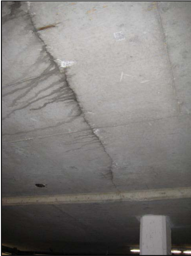
Photo No. 5: Underside of P! Level Suspended Floor Slab Note: Crack in concrete with evidence of leakage.
