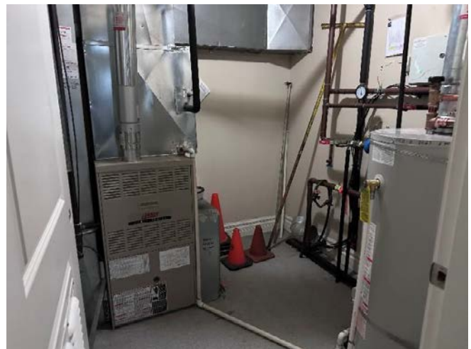
Photo 12. Mechanical room at the Amenity Building.
