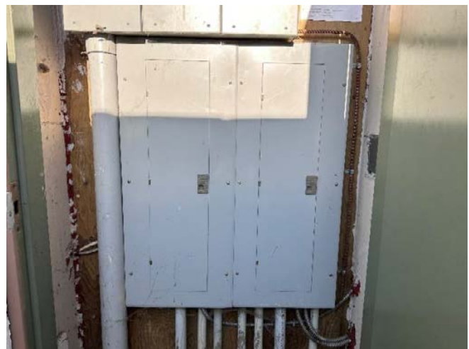
Photo 48. View of the electrical panels located at the south side of Amenity Building.
