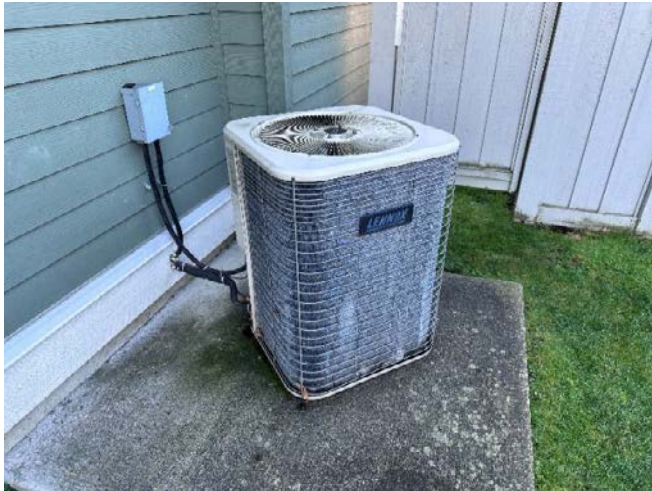
Photo 19. Air Conditioner condenser unit at the exterior of the Amenity Building.
