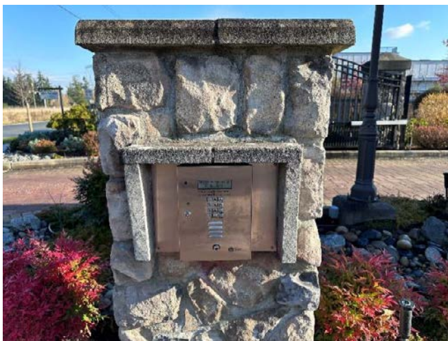
Photo 41. View of the communicator panel at the main front gate entry.
