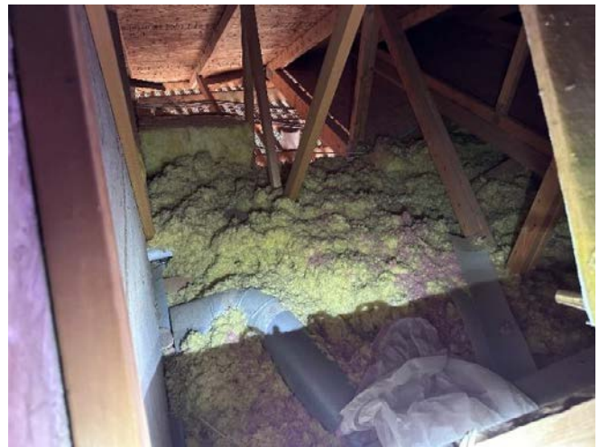
Photo 4. Example view of an attic space with exposed ducting and poor distribution of the attic insulation.
