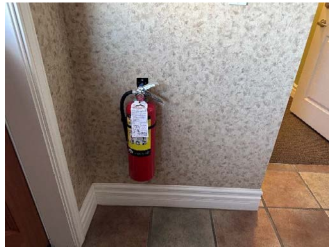
Photo 16. Fire extinguisher at the Amenity Building.
