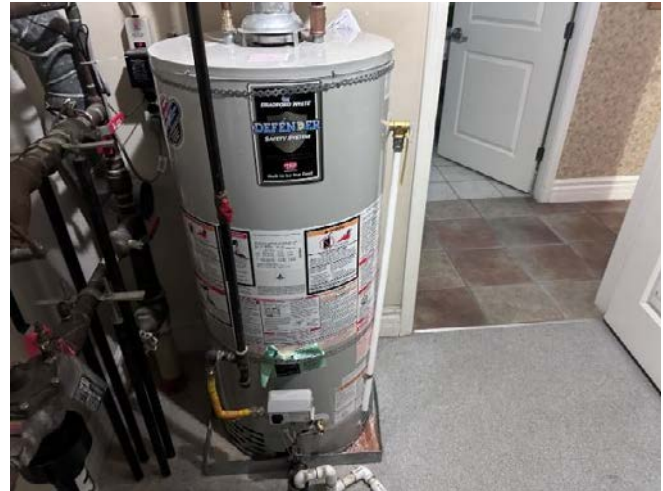
Photo 14. Domestic hot water heater at the Amenity Building.
