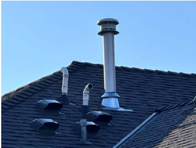
Photo 31. Example view of the metal chimney, furnace exhaust, fresh air pipes, and exhaust vents.
