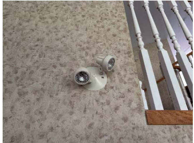
Photo 8. Emergency lighting at the Amenity Building.
