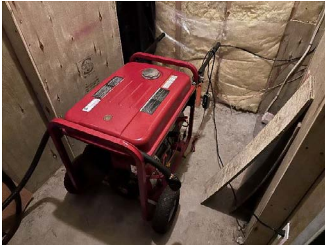
Photo 43. Emergency generator at the gate house.
