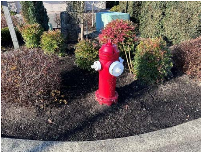
Photo 29. Fire hydrant along the roadway.
