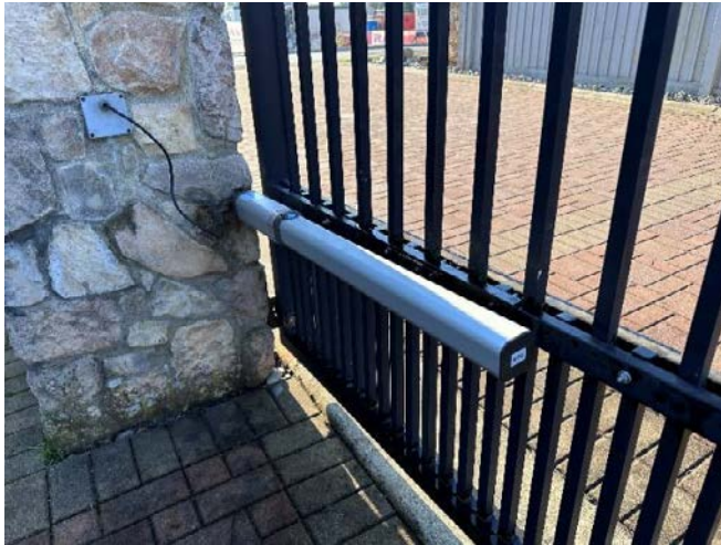
Photo 25. View of an automatic gate opener.
