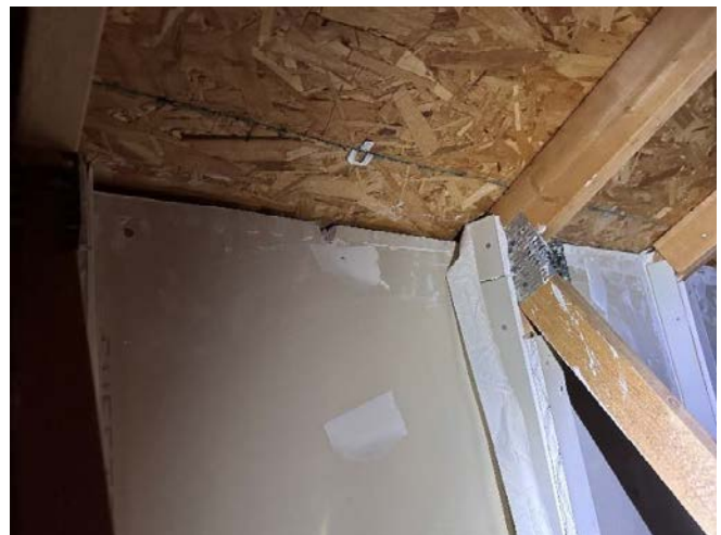
Photo 6. Example of the separated drywall joints at a sample attic.
