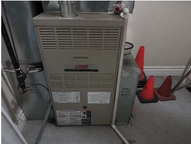
Photo 13. Gas-fired furnace at the Amenity Building.
