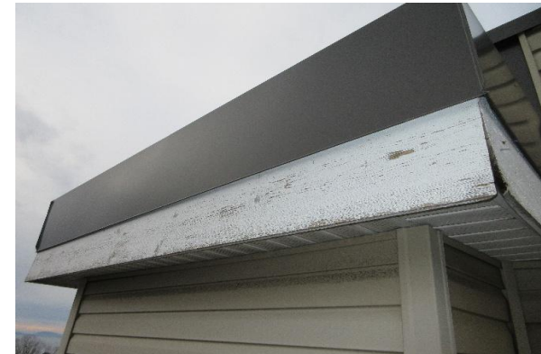
Peeling paint on wooden fascia boards
