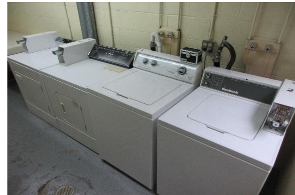
Washing and drying machines
