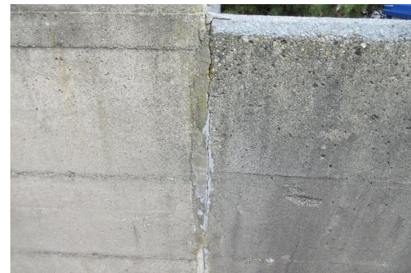
Cracks in concrete wall at the cold joint
