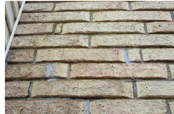
Cracks in brick veneer mortar joints and units
