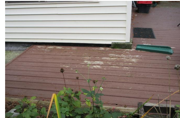
Peeling paint on wooden patio decking
