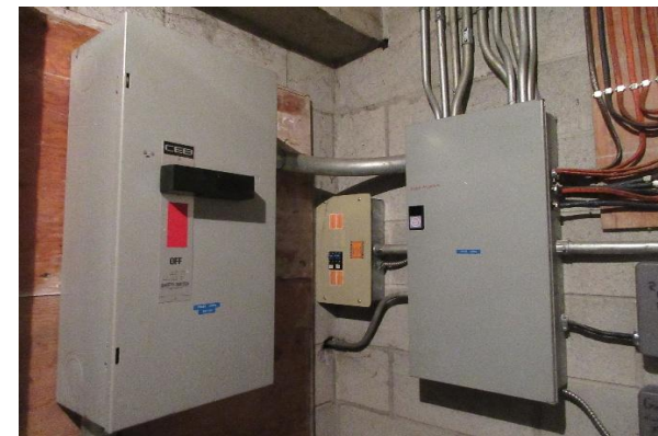
Electrical switches and panels
