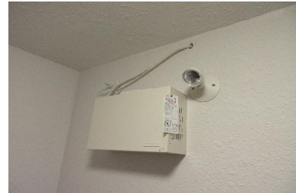
Emergency light with battery pack
