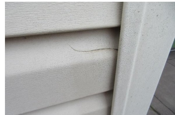
Crack in vinyl lapboard siding
