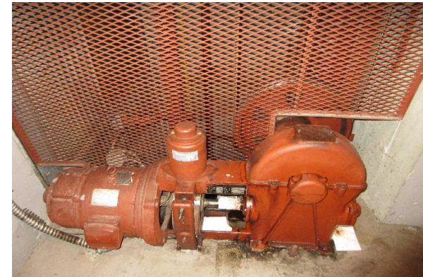
Hydraulic elevator machinery
