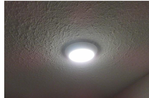
Interior ceiling-mounted light fixture
