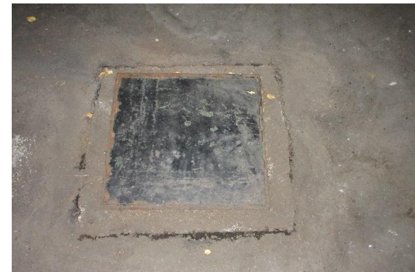
Sump tank cover
