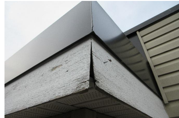
Warped and separated wooden fascia boards
