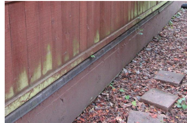
Paint on concrete wall below wooden fencing
