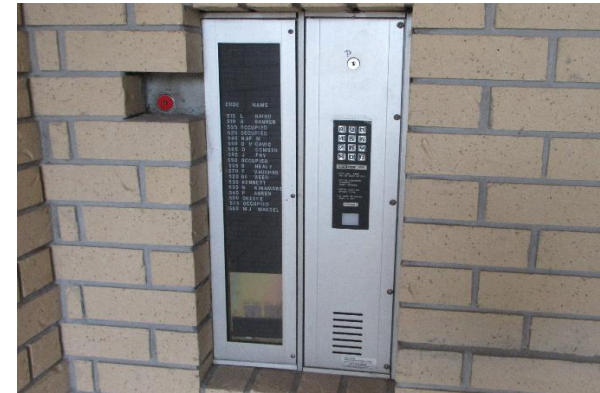
Access control panel
