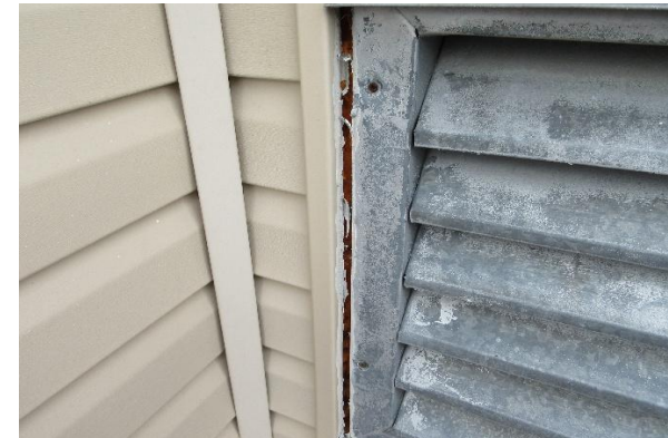
Failed caulking at vent penetration
