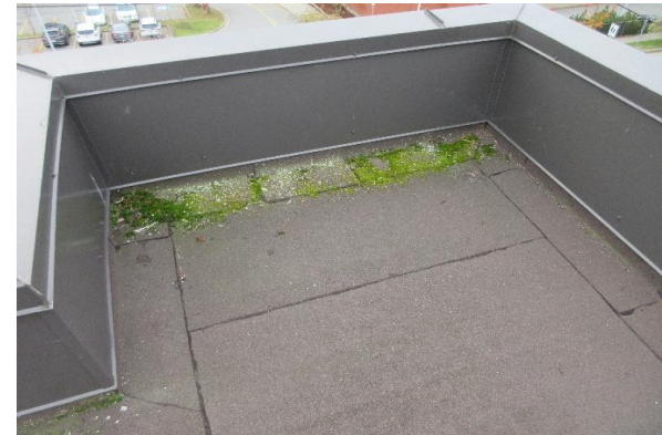
Moss growth on SBS membrane roofing
