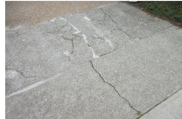
Cracks in concrete paving
