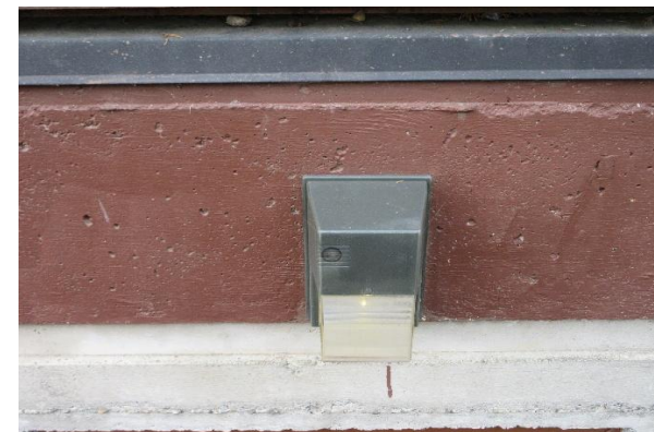
Exterior facade-mounted light fixture
