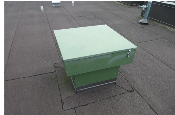
Make-up air unit
