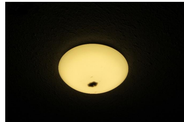
Interior ceiling-mounted light fixture
