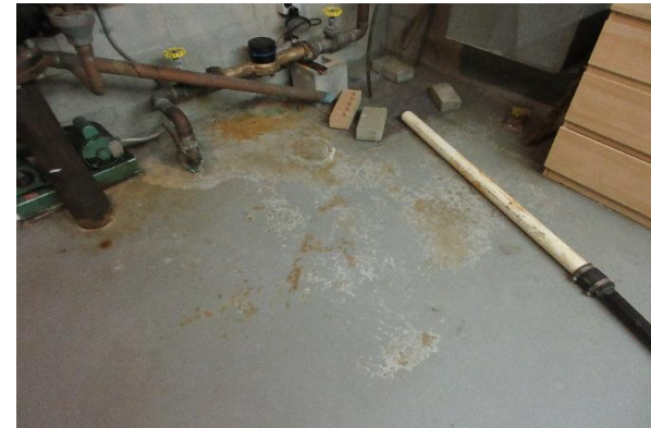
Stained traffic coating
