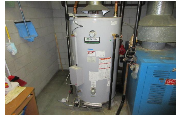
Hot water heater
