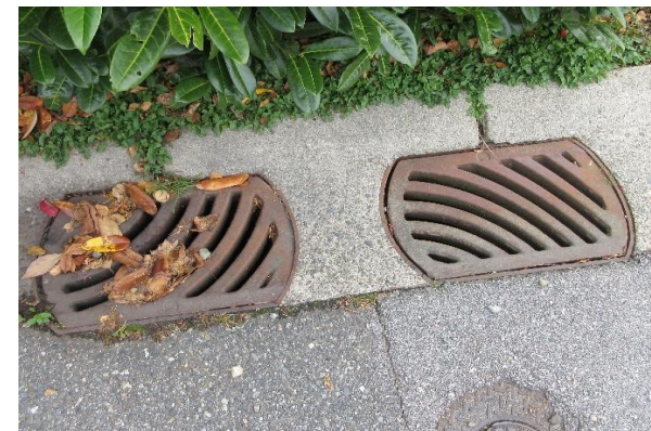
Storm catch basins
