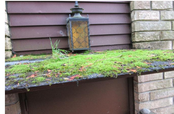
Moss growth on asphalt shingle overhang
