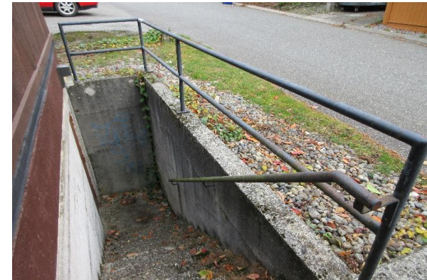
Corrosion on exterior aluminum railings
