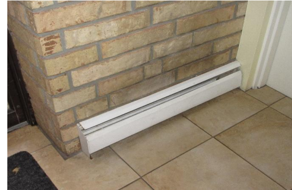
Electric baseboard heater
