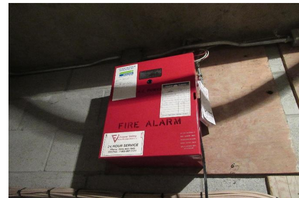
Fire alarm system
