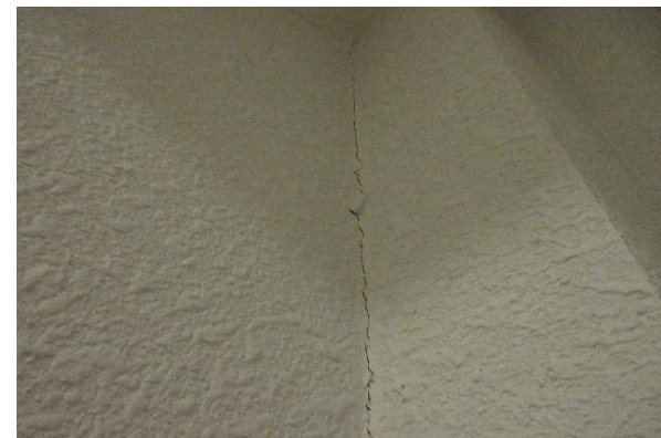
Cracks in wall finishes
