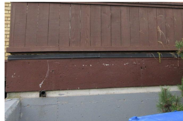
Paint on concrete wall below wooden fencing
