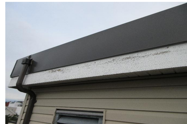
Peeling paint on wooden fascia boards
