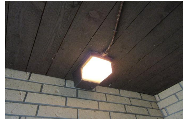
Exterior soffit-mounted light fixture
