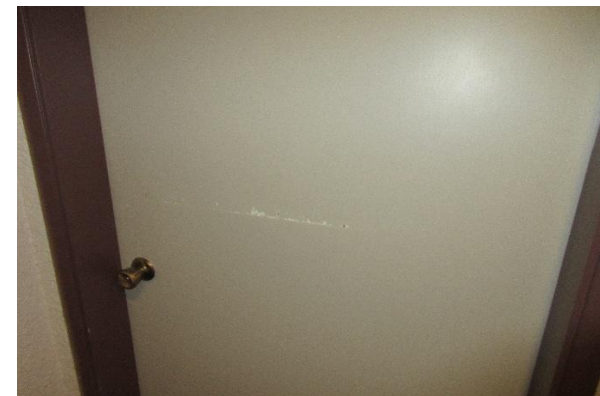
Peeling paint on wooden unit entry door
