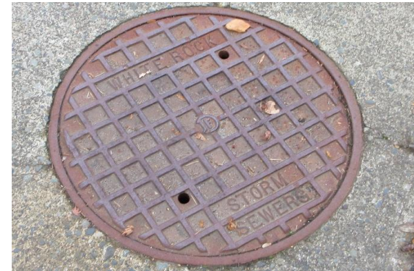
Storm manhole cover
