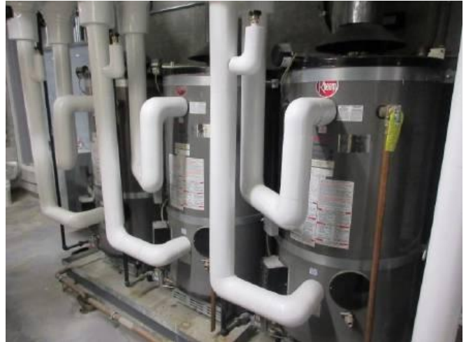
Photo 34: Typical water heaters.
