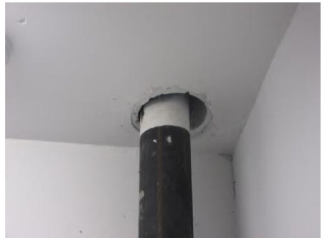
Photo 16: Standpipe slab penetration without firestopping.
