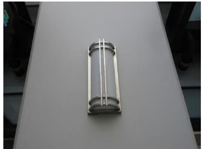
Photo 40: Typical exterior wall sconce.
