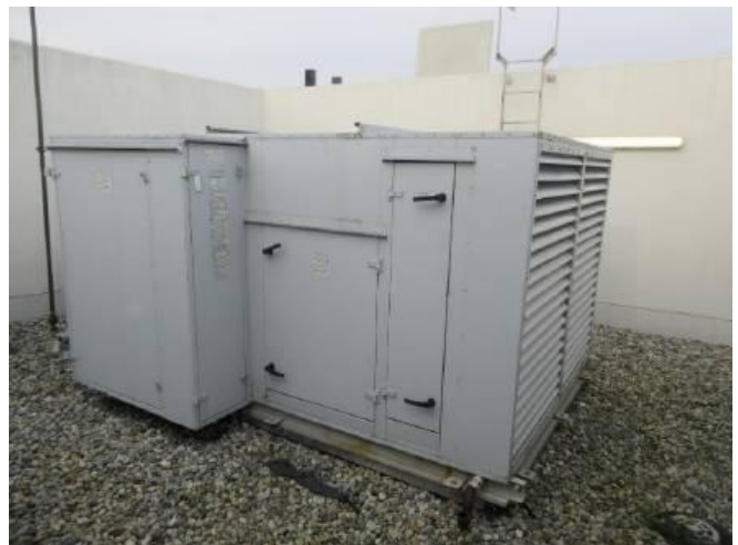
Photo 32: Typical heating boiler.
