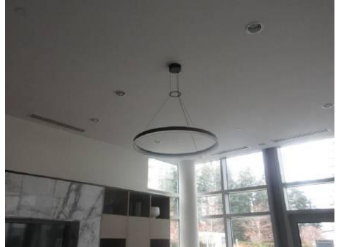
Photo 39: Lounge pot lights and ceiling mounted fixture.
