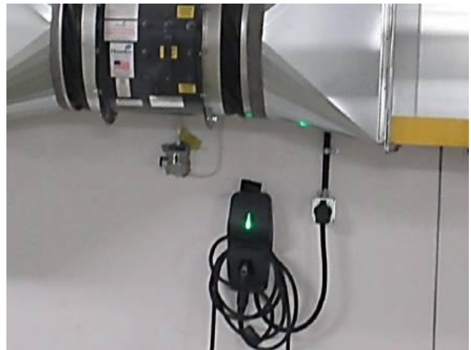
Photo 38: Electrical vehicle charging station.
