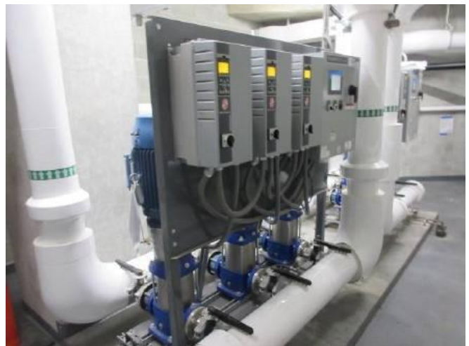
Photo 35: Typical booster pump set.
