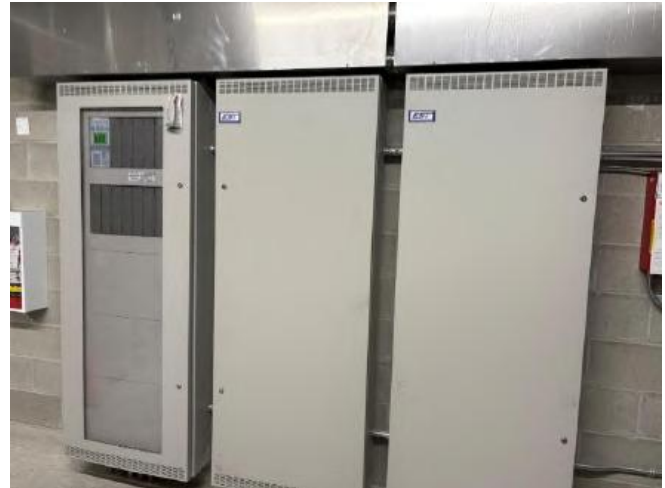
Photo 17: Fire alarm control panel.
