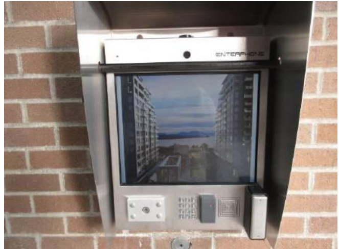
Photo 45: Typical tower entrance enterphone panel.
