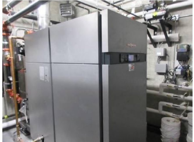
Photo 31: Typical heating boiler.
