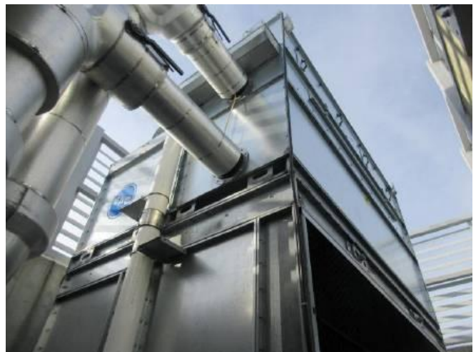
Photo 33: Typical cooling tower.
