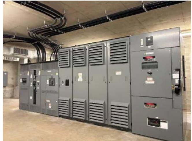
Photo 37: Incoming electrical equipment.
