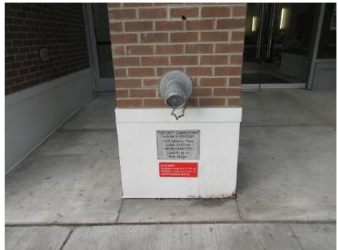
Photo 20: Fire department connection.
