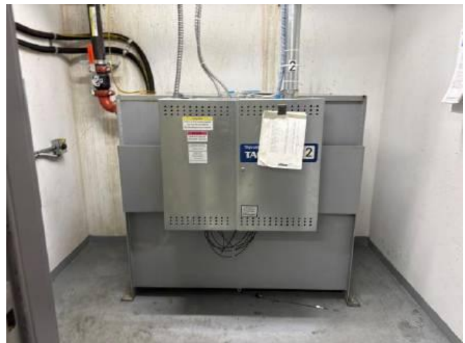
Photo 42: Hydraulic elevator equipment.
