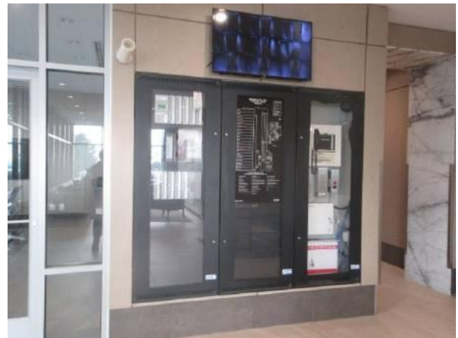
Photo 18: Typical annunciator panel.
