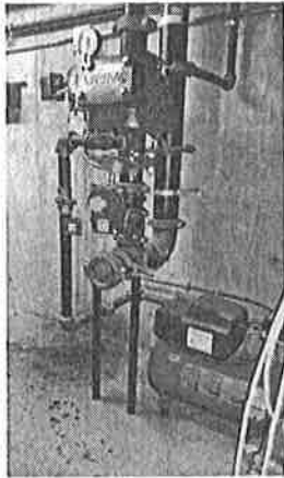
(33) – Sprinkler Tree for Parking Dry System
