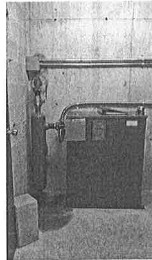
(45) – Elevator Machine Room Hydraulics
