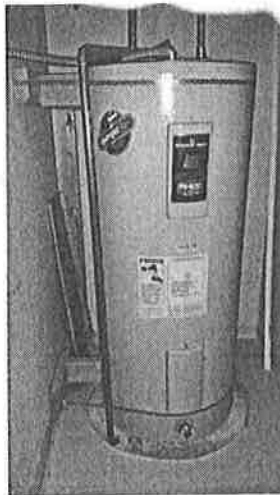
(39) - Individual Electrical Hot Water Tanks (Bradford White)
