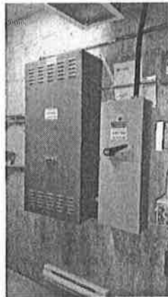
(44) – Elevator Electrical Panel
