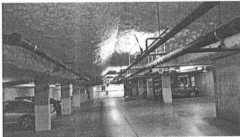
(36) – Sprinkler Distribution in Parkade
