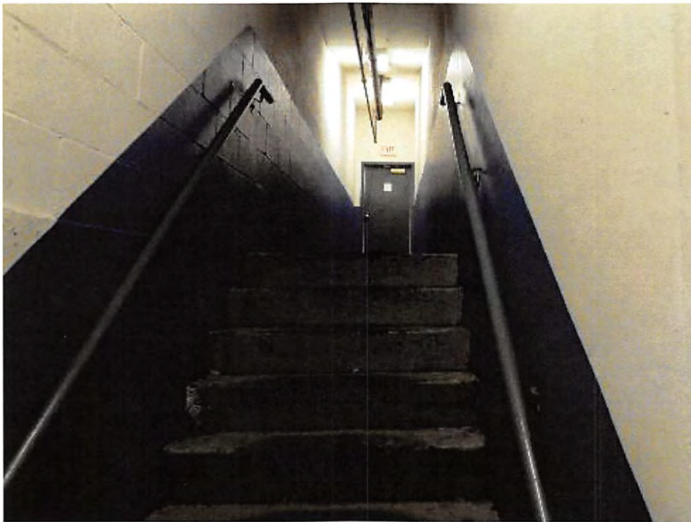
Cracking in stairs
