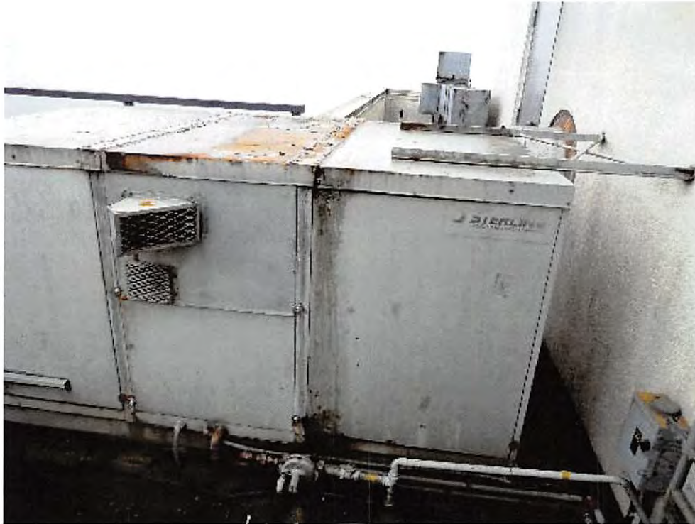
Make-up air unit
