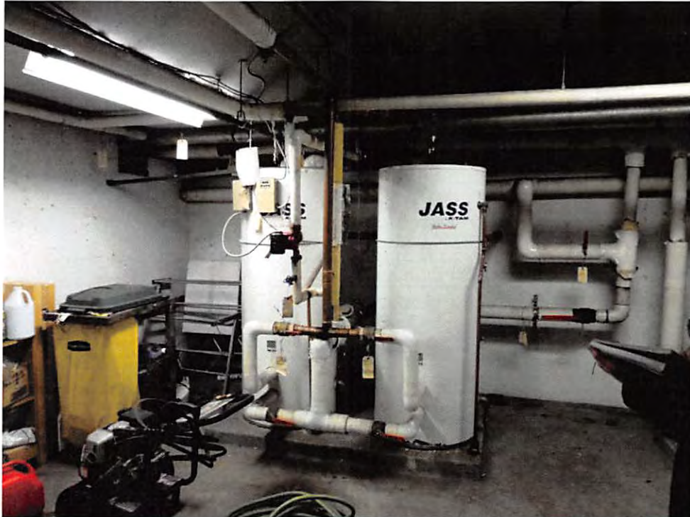
Hot water tanks
