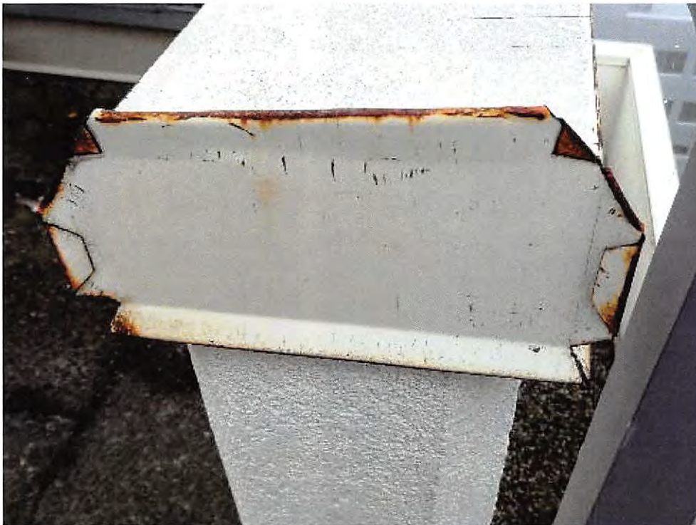
Rusty flashing on parapet wall
