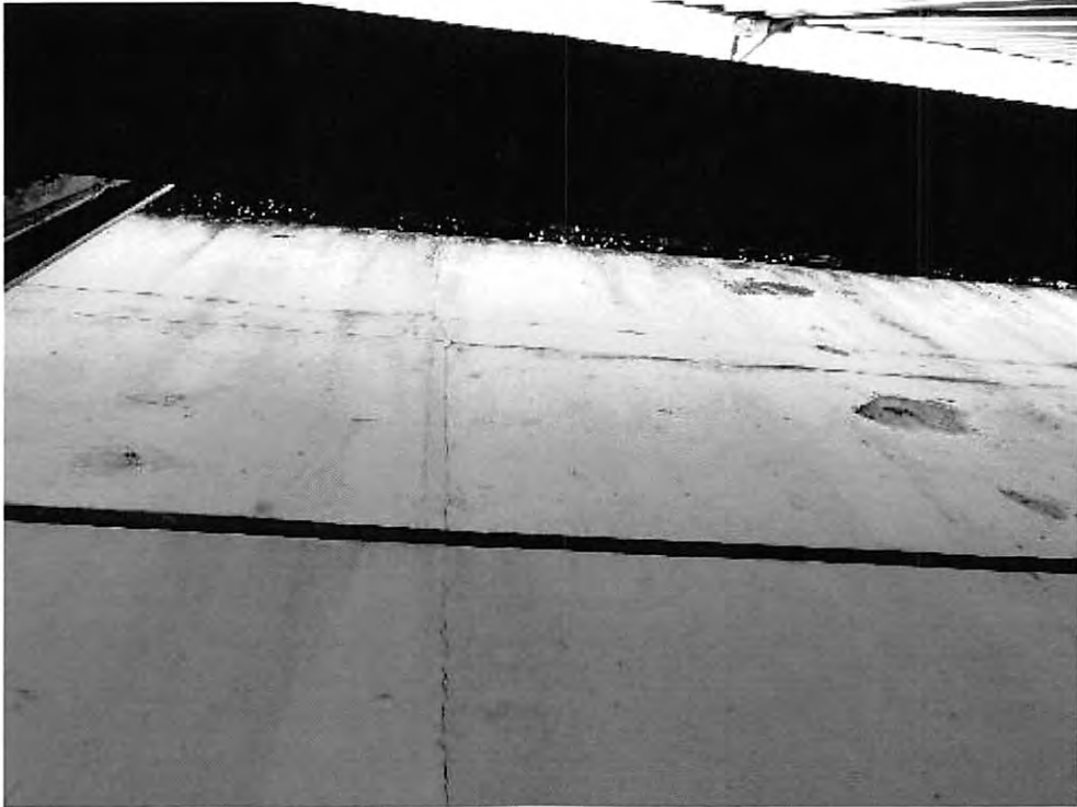
Paint deterioration on building exterior
