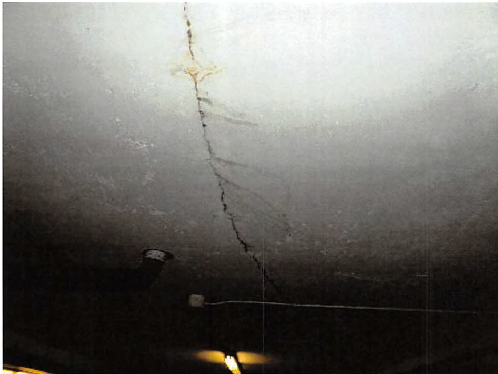
Leaky cracks in ceiling
