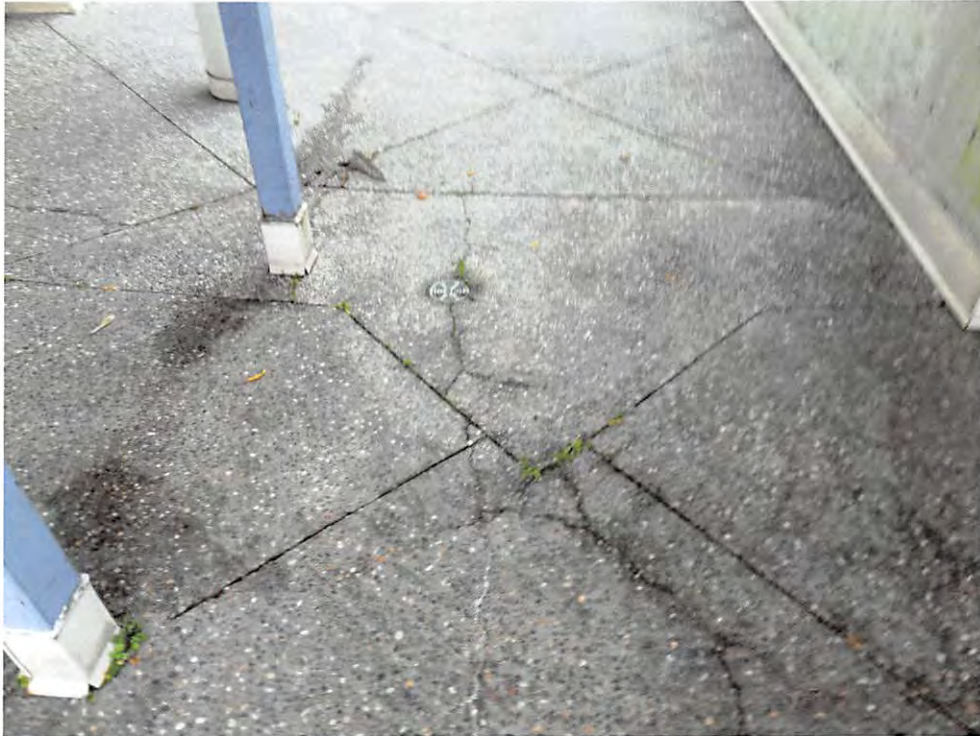
Cracks in concrete pavers
