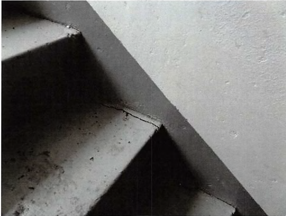
Cracks in stairs
