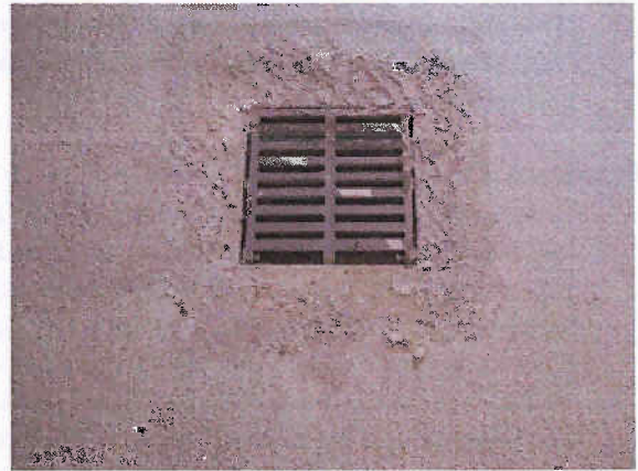
Photo 2.5.4: Urethane traffic membrane delaminated around the perimeter of a drive aisles drain.
