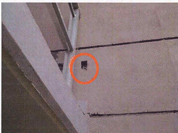
Photo 2.1.12: Electrical box installed 4" beyond the outer face of the balcony railing at Unit 2406.
