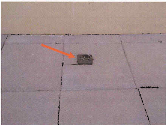
Photo 2.3.3: Bi-level drain extends above the finished walking surface at the level four plaza deck.
