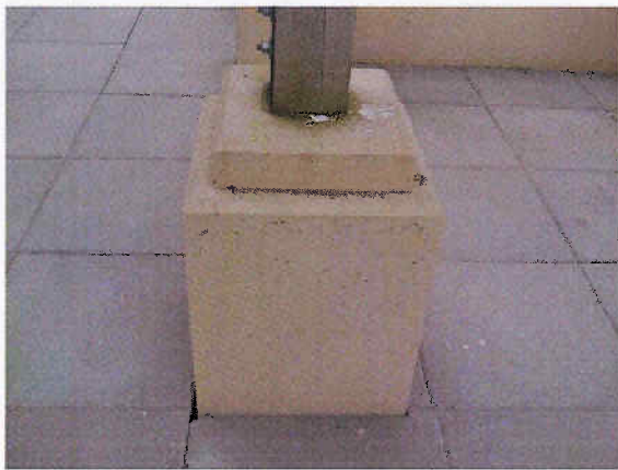
Photo 2.1.7: Pock marks with bare concrete visible at a concrete pedestal on the level four plaza deck.
