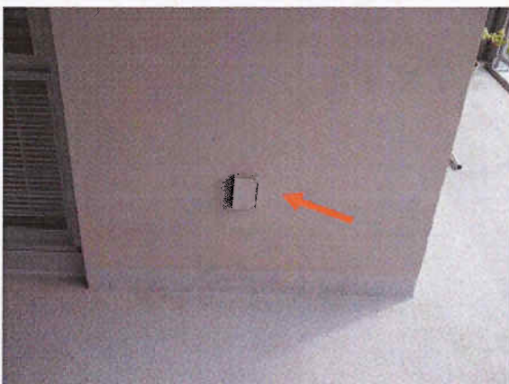
Photo 2.1.11: Typical exterior electrical box outlet.
