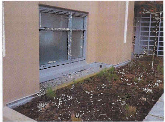
Photo 2.5.2: Gravel trench and gum-lip flashing installed at a planter building wall intersection.
