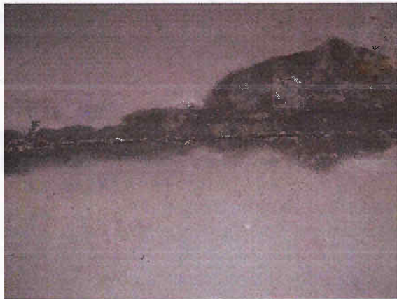
Photo 2.5.3: Water ingress at the base of the concrete wall sub-grade slab intersection at parking stall 59.
