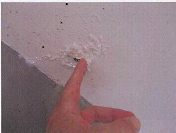
Photo 2.1.5: Efflorescence stains at the underside of the balcony soffit above Unit 506.
