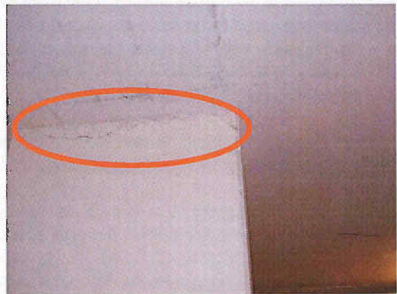
Photo 2.5.6: Delaminated concrete at the top of the column north of parking stall 63.
