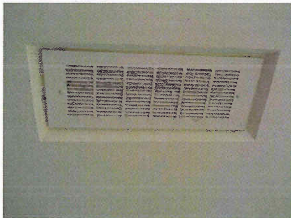
Photo 2.1.10: Louvered dryer exhaust vent grill partially clogged with lint.
