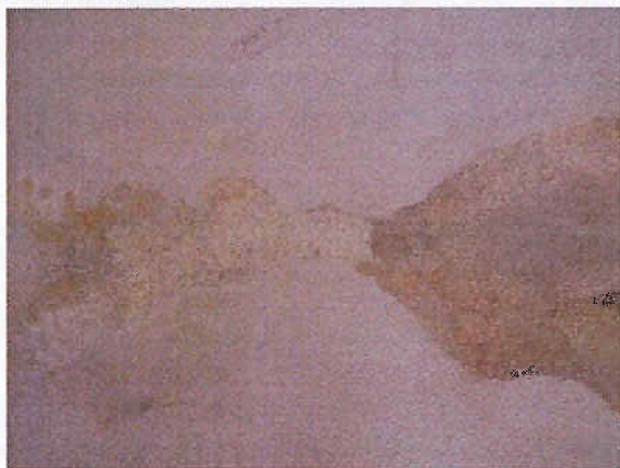
Photo 2.5.5: Urethane traffic membrane delaminated at the drive aisle south of parking stall 156.
