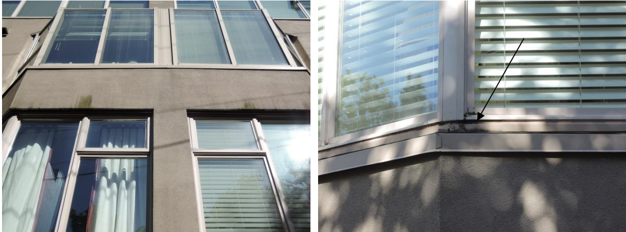
Fig 27 - East face sealed window and wall assembly with moss and algae growth on stucco above bay windows (left). Algae and mildew are clearly visible on window sill flashings (arrow at right).
