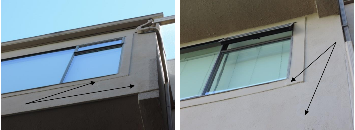
Fig 21 – South facing window installation - the absence of head and sill flashings and the age of the sealants both reduce the ability of the windows to shed water. The window shown on the right has some overhang protection but this is not preventing deterioration of the wall surface as indicated by the cracks (at arrows).
