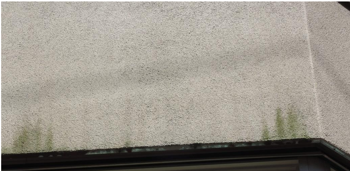
Fig 12 – Close-up of moss and algae growth on a stucco surface. Notice the rust at the metal base flashing.
