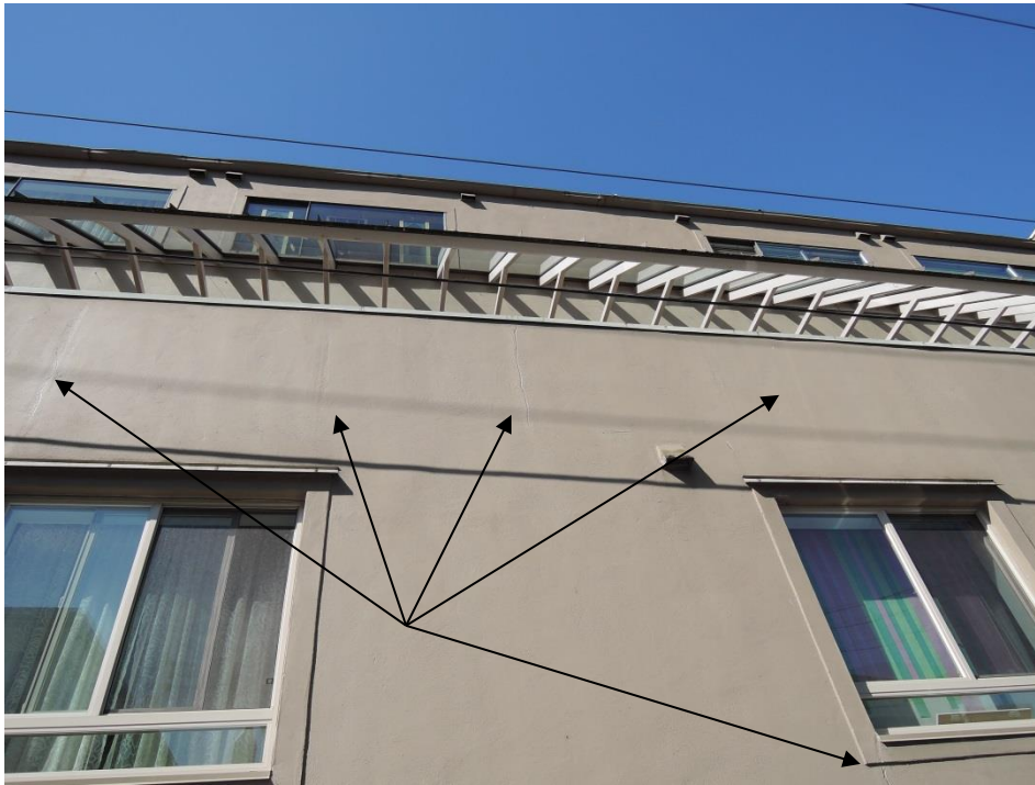
Fig 4 – Cracks run vertically above windows on the parapet wall as well as at the corner of windows.
