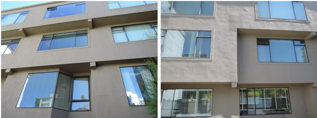
Fig 9 - Stucco surfaces around units 105- 108 and 304-308. Old style windows and face sealed windows installed in a standard cladding system.
