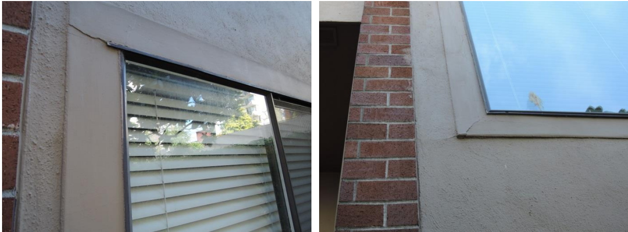
Fig 25 – Original window installation at the southwest face (left). Lack of caulking at this area is resulting in cracking and water penetration. These windows are of similar design and age of those on the south face of the building and also have extensive areas of stucco.
