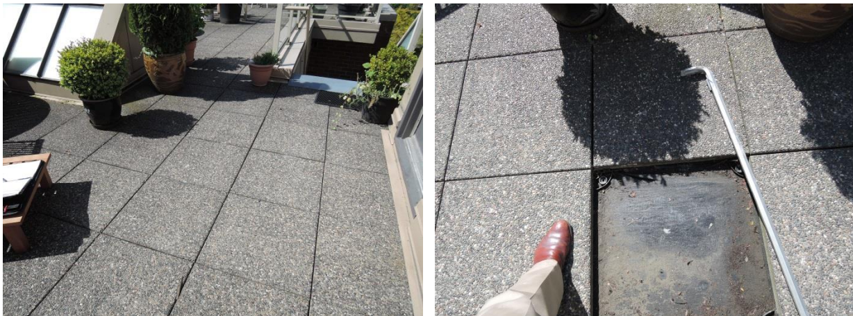
Fig 28 – Paved roof deck area and stairwell access to a single unit (left). The filter cloth membrane visible under pavers (right).
