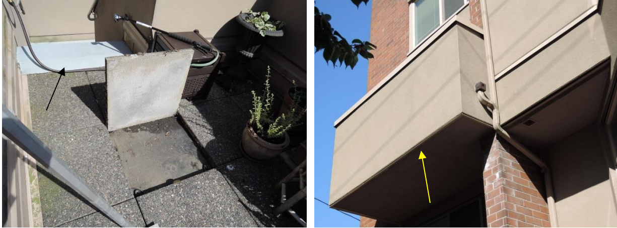
Fig 31 - NW stairway has water ingress (left) and watering of planters may be the cause. Leachate is visible on the underside of this balcony (right).
