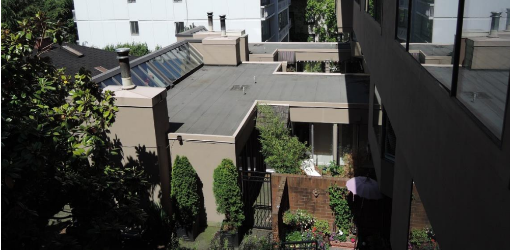
Fig 2 – View of two single story units (104,106) and the flat roof above them.
