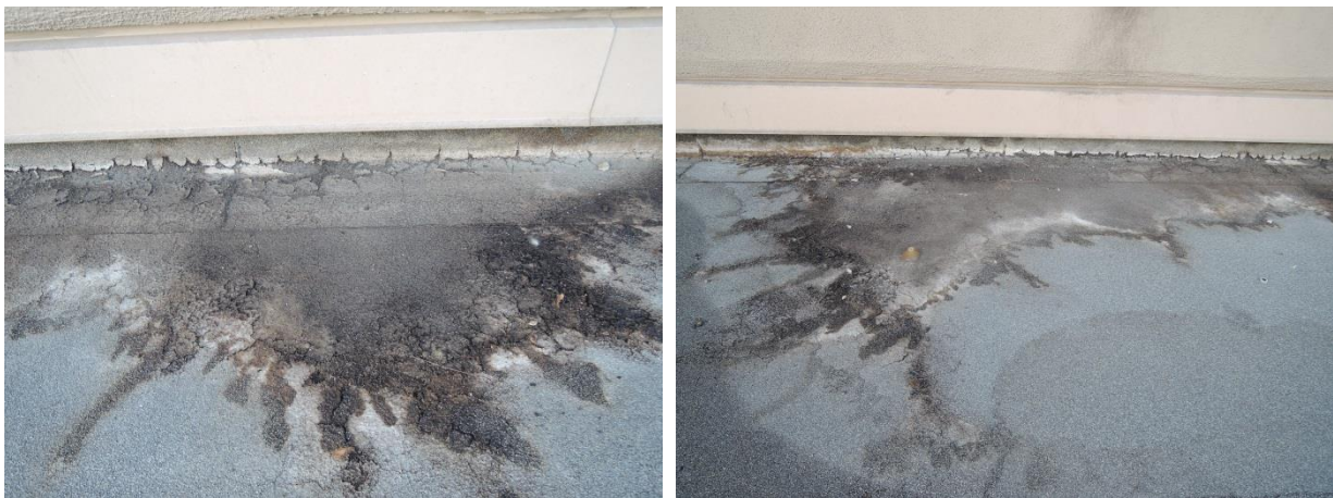
Fig 33 - Large area of staining and deterioration of flat roof surface.
