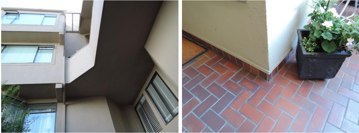
Fig 15 – South face to the left and west face to the right. Stucco terminated at tile and flashing on the west face (right).
