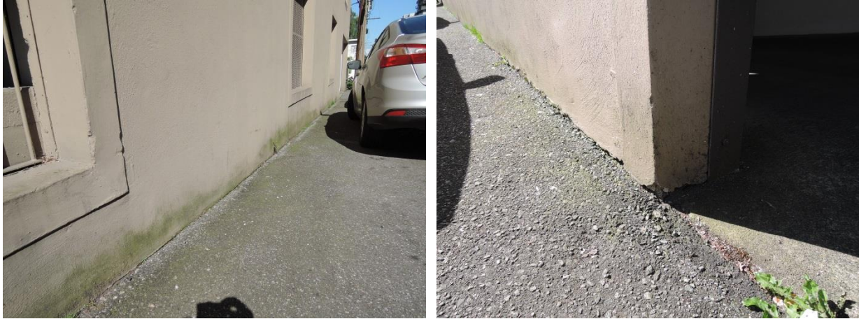
Fig 6 - There is no drip screed at the base of this wall resulting in moisture penetration as indicated by the presence of moss and algae growth (left). The stucco surface terminates at the asphalt surface of the lane (right).
