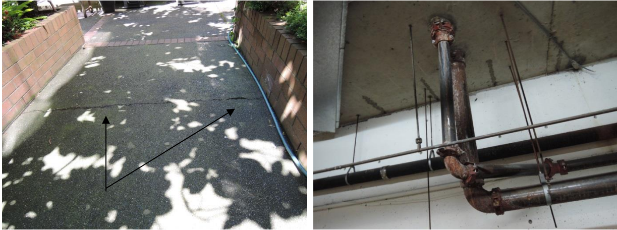
Fig 40 – Crack in walkway (arrows left) and rusting metal drainage pipes (right).
