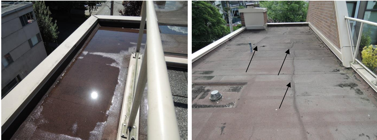
Fig 34 - NE flat roof has poor drainage (left) and long ridges in the membrane (at arrows right).
