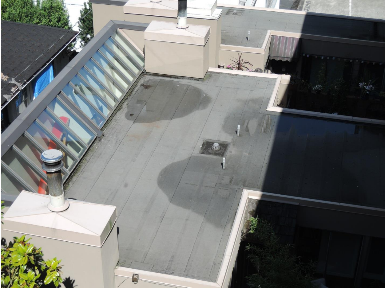
Fig 32 - Flat roof over units 106 and 104. Note the ponding water at several locations.
