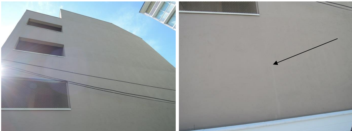
Fig 5 – Large areas of stucco have no control joints or stress relief mechanisms to prevent cracks caused by thermal movement (left). Caulked cracks are the result of thermal movement in these areas (right).
