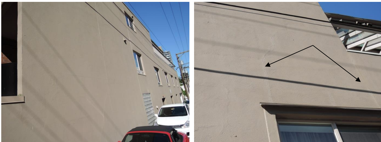
Fig 3 – The North face is shown (left). This large area of stucco has no provision to deal with thermal movement. Caulked cracks above a window and at steps in the wall surface (arrows at right).
