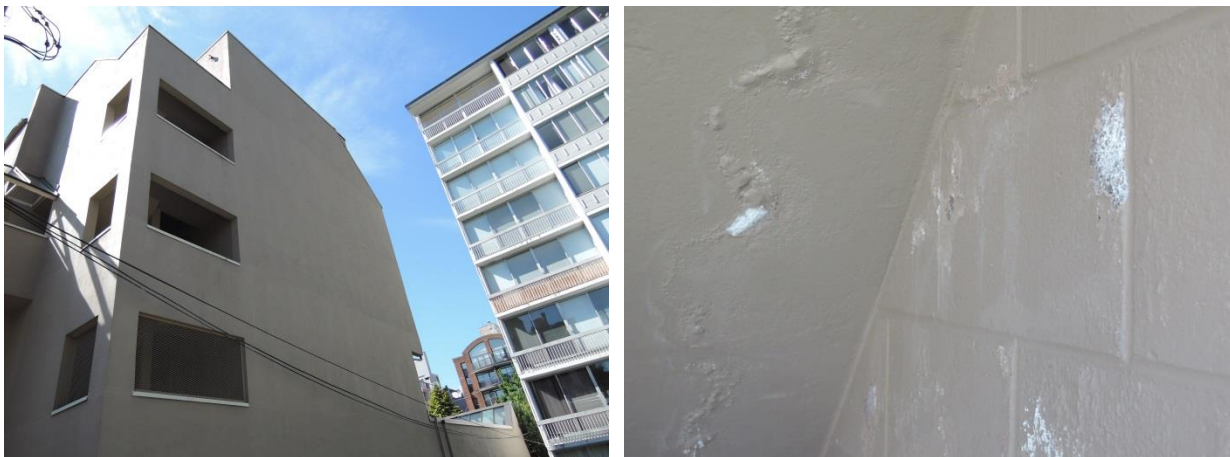
Fig 30 –NW face stairway (left) and efflorescence in concrete blocks coupled with high moisture readings indicate water is penetrating and migrating through the blocks to the surface (right).
