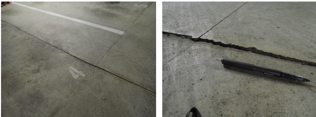
Fig 41 - Differential settlement crack location (left) and close-up view with 6 inch pen to indicate scale (right).
