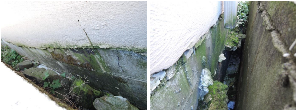
Fig 7 – Poor stucco termination and finish and the absence of drip screed (left). Downspout discharge and poor drainage arrangement further compounding water ingress potential (right).
