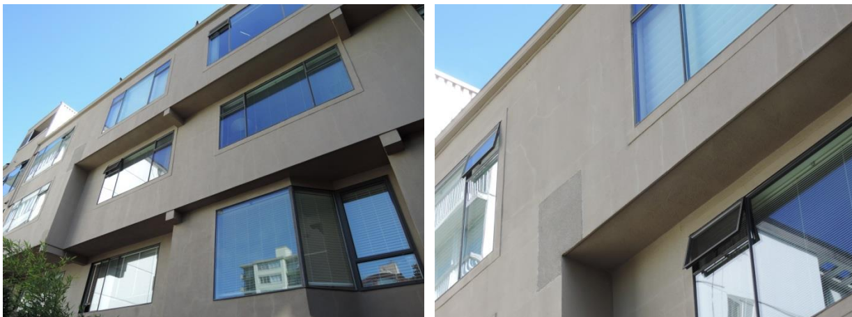
Fig 20 - South face (Units 105 -108 1 st floor and Units 304 -308 3 rd floor) showing original windows and stucco wall cladding (left). A patch from the 2000 BECA is shown in close-up (right). Notice the large number of streaks in the stucco face – this is an indication of moisture in the wall assembly.
