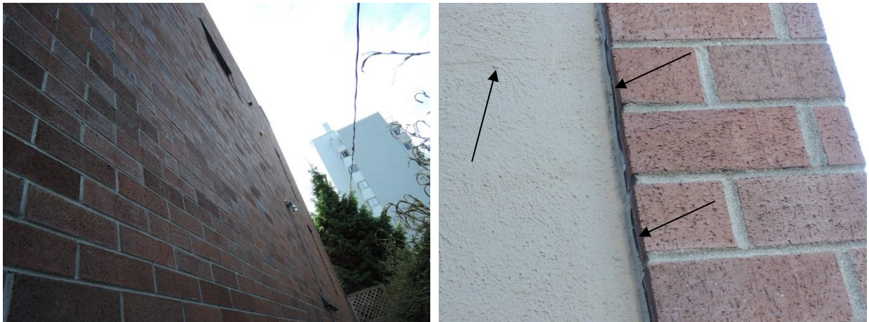
Fig 14 - Brick veneer on the south face (left). Transition caulking deficiency and stucco crack (arrows at right).
