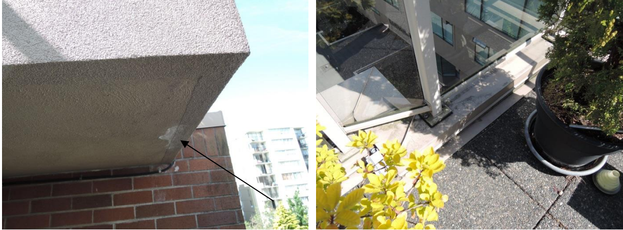
Fig 29 -leachate from roof deck above (left) and surface above the leachate point (right).
