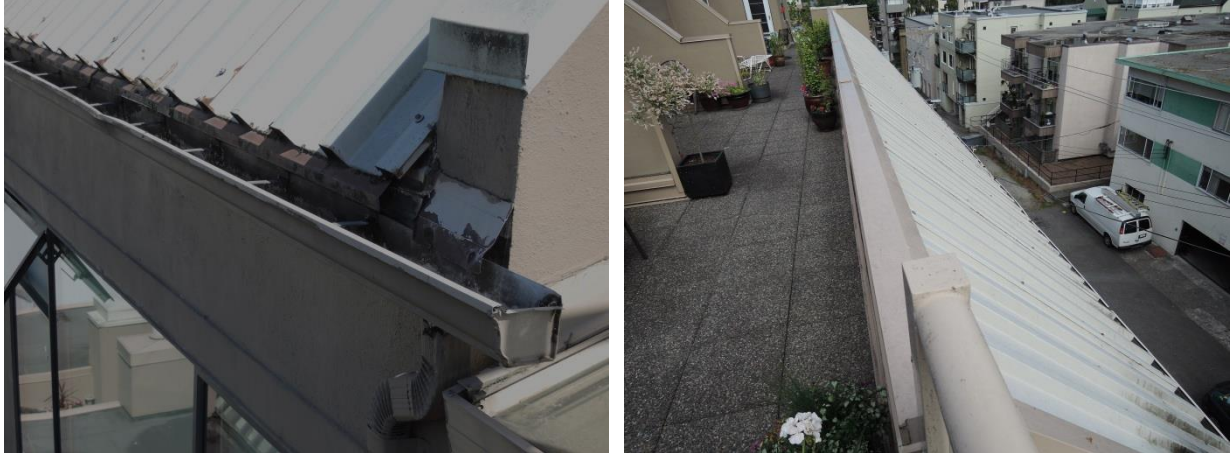
Fig 36 - There are some minor areas of rust on the sheet metal roofing.
