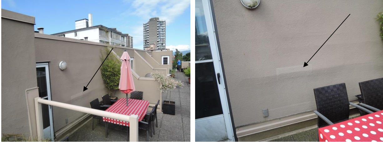
Fig 8 - North facing roof deck with 4 units. The strata has repaired the cracks (at arrows) of the ballooning surface and have also replaced the wall surface of the third unit (306).
