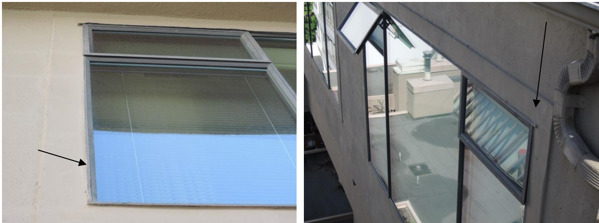
Fig 22 - Poor condition of the caulking between the window frame and wall (left). Stucco accent or reveal with cracks and old style head flashing detail (right).
