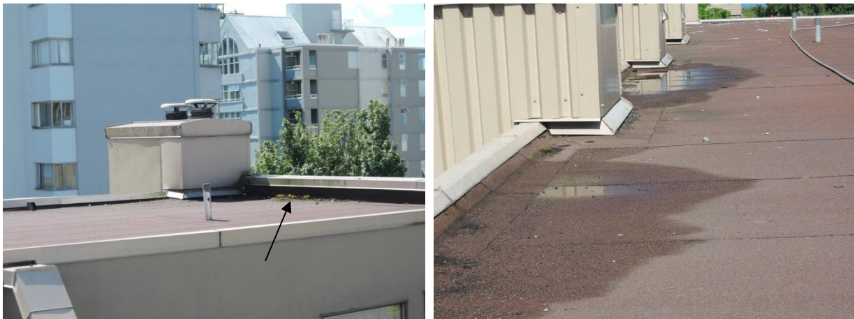
Fig 35 – Moss and algae growth adjacent to SE chimney (arrow left) and minor ponding on the flat roof (right).
