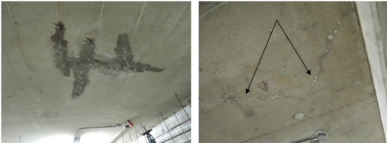
Fig 39 - Epoxy repair to overhead slab (left) and minor shrinkage crack and leachate (arrows, right).
