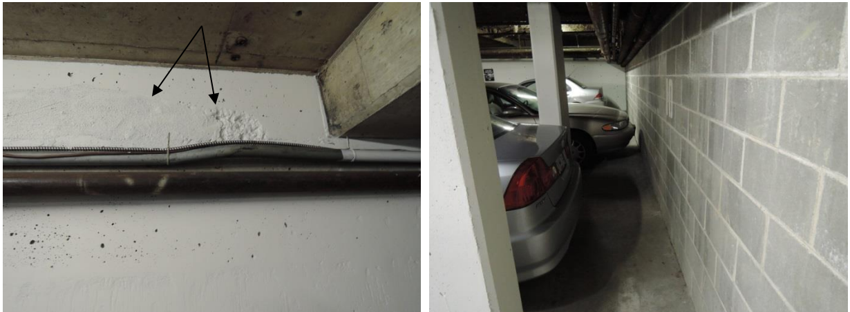
Fig 37 - Foundation wall repair (left at arrows) and the condition of concrete block foundation (right).
