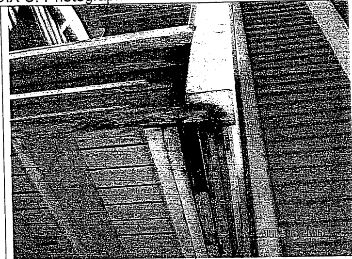
4- Original drip type deck showing rot at out side corner
