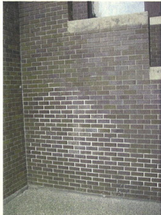
Photo 08 Efflorescence on the exterior stairwell
