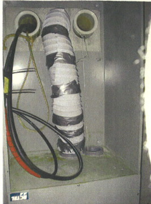
Photo 34 Water ingress at the Telus cable box in the bike storage room
