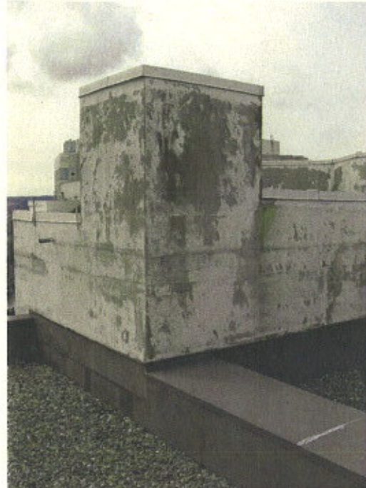
Photo 14 Erosion of the paint on concrete and inadequate saddle detail
