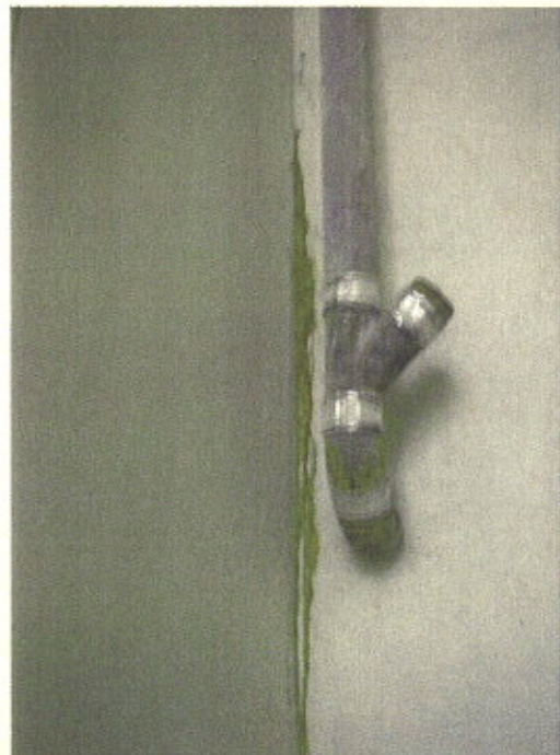
Photo 40 Dark staining on the wall adjacent to the planter
