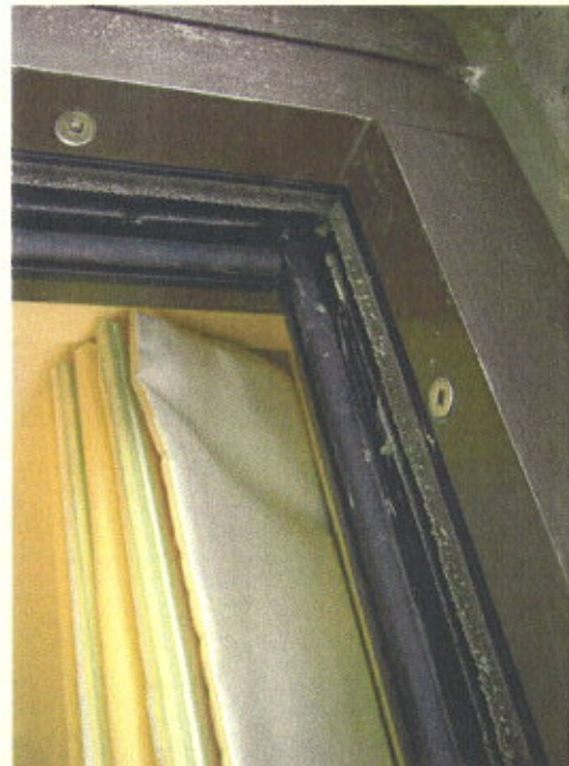
Photo 20 Inadequate gasket at the door
