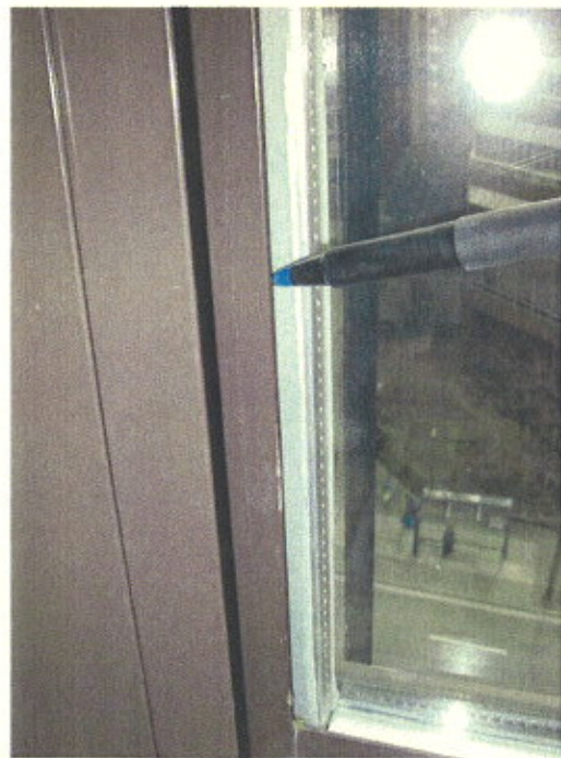
Photo 24 Displaced aluminum spacer in unit 1008
