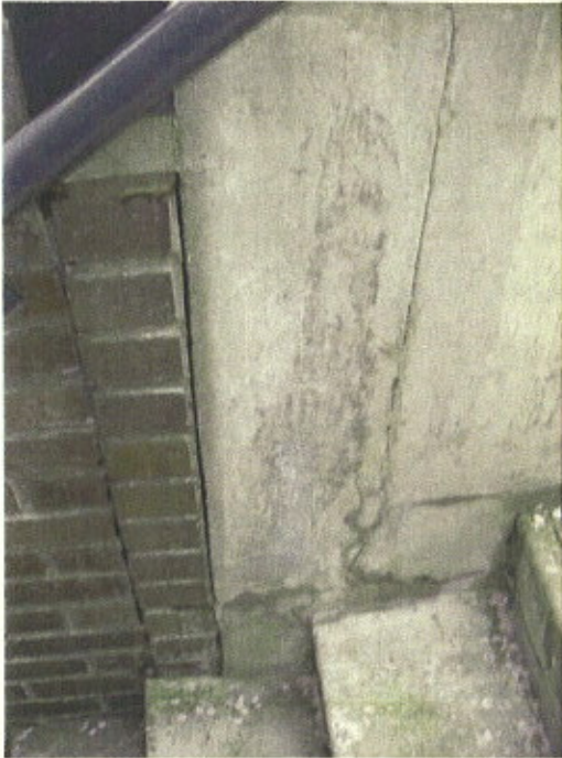
Photo 09 Open joint between concrete wall and masonry
