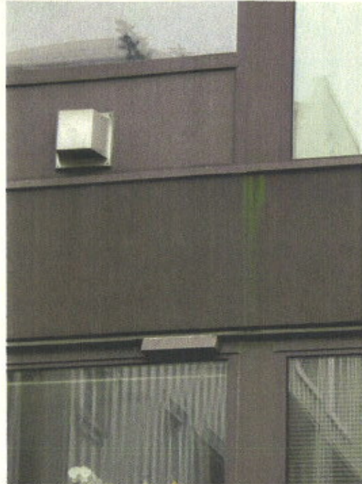
Photo 18 Modified hood over the exhaust vent
