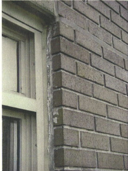
Photo 06 Efflorescence at the door and brick transition. Shortened gasket in the spandrel
