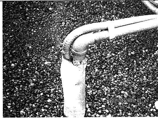
Photo 30: Another HVAC service vent that requires sealing.
