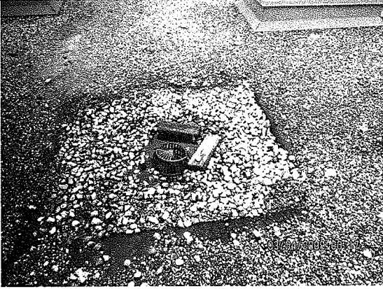
Photo 13: Drain sump on 2983. The edges of these sumps can be one of the first areas to show deterioration. This one appears to have been repaired in the not too distant past.
