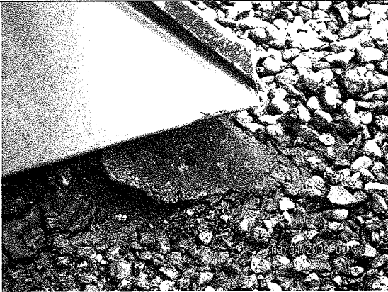
Photo 26: Another example of deterioration of the membrane at the curb.
