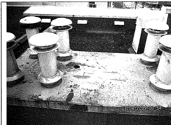
Photo 23: Here we have a chase cap that is beginning to rust. Any rusting flashings should be cleaned and give a fresh coat of rust resistant paint.
