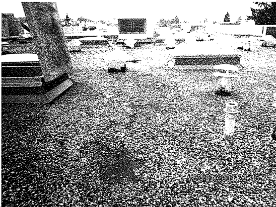
Photo 2: Photo showing buckles and blisters that have been covered with SBS membrane.
