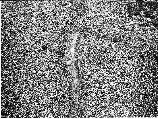
Photo 18: Another example of a buckle that should be repaired.
