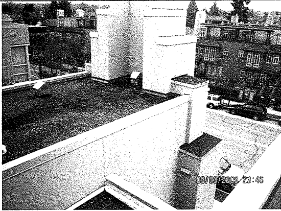
Photo 6: Lower roof at front of building. When reroofing is undertaken, the stucco in these locations will need to be cut back to allow the new membrane to extend up the walls a sufficient height.
