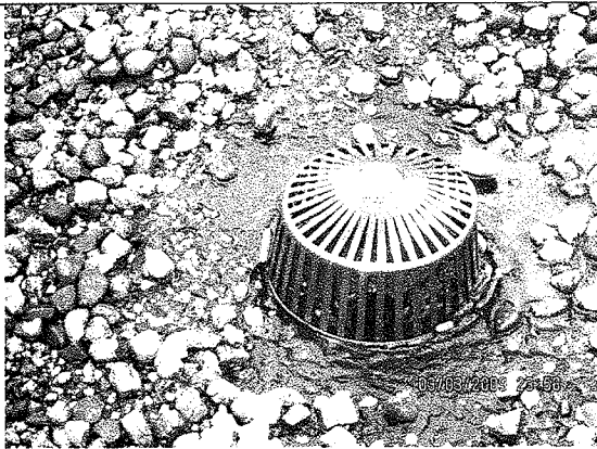
Photo 7: Here we have a drain that has obviously been leaking. Although this seems to have done the job, a more permanent solution would be to add an SBS patch over the area.
