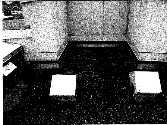
Photo 34: This photo shows build up of moss on roof at front of building. This should be removed, as it has a tendency to hold moisture in the area, which can cause premature deterioration. It also shows how the stucco has been cut back during the rainscreen process. This should help when it comes time to replace the existing roof.
