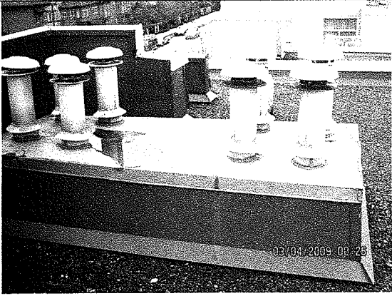
Photo 17: Chase cap that is not shedding water as it should. This should be corrected so that chase cap does not rust prematurely.
