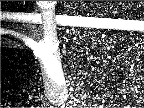
Photo 4: Gas and electricity service for HVAC unit with mastic showing signs of cracking. These should be properly sealed.
