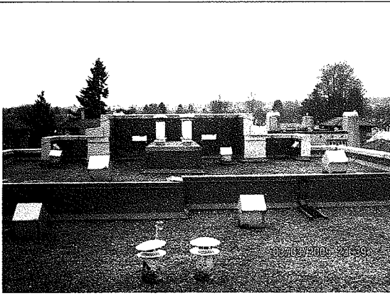
Photo 1: Raised roof area with metal flashing on parapets. When roofs are changed, these walls should be covered with 2 ply SBS membrane.
