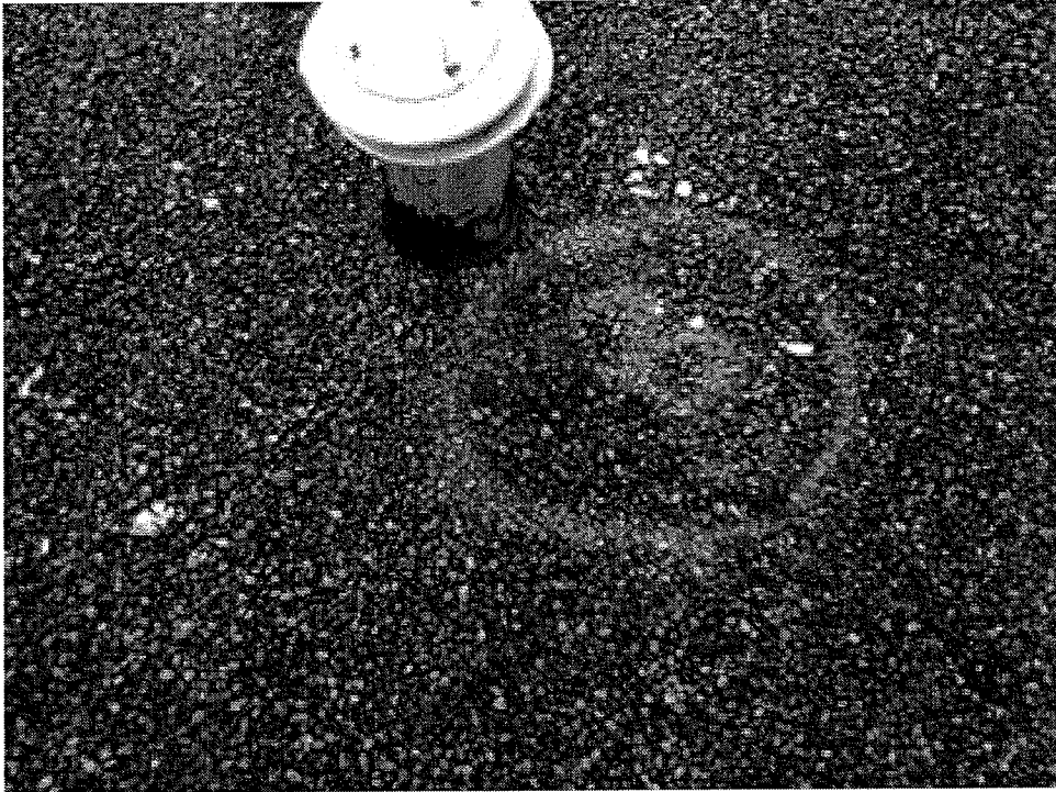
typical blister east roof
