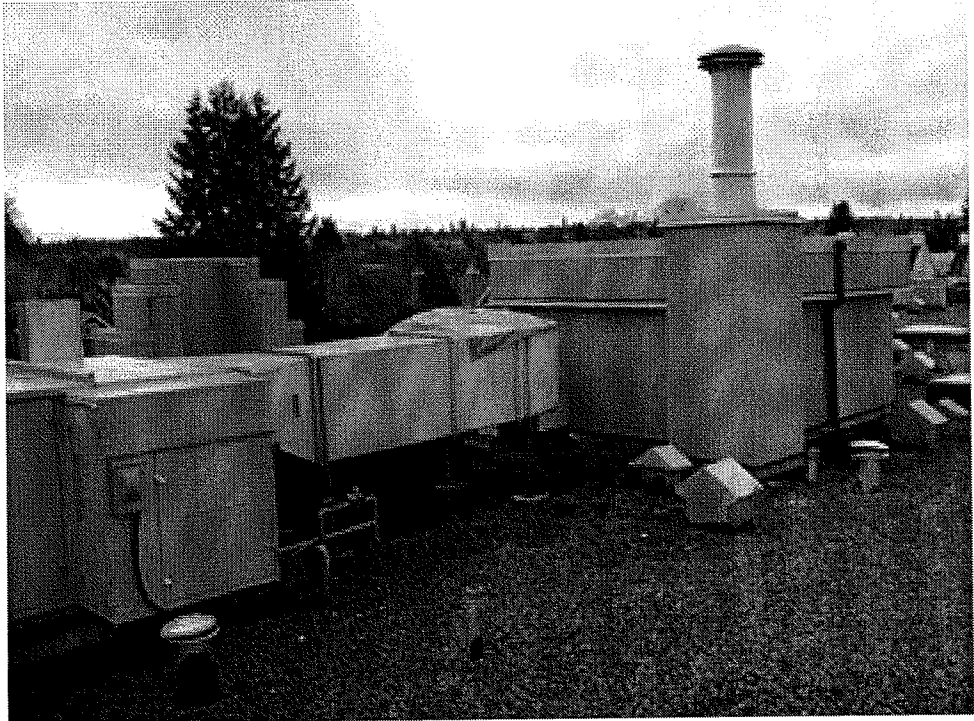
tarped unit on west roof
