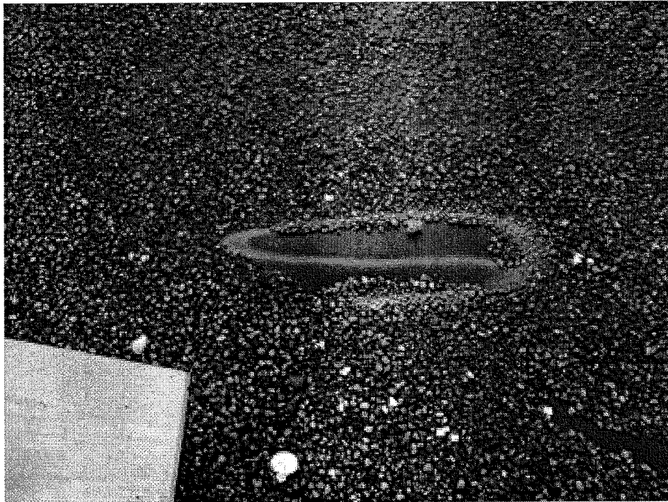
old repair failed
